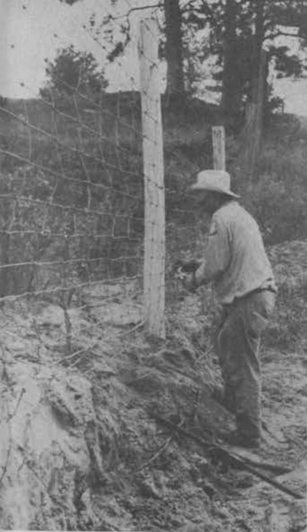
Fence maintenance is a routine chore
