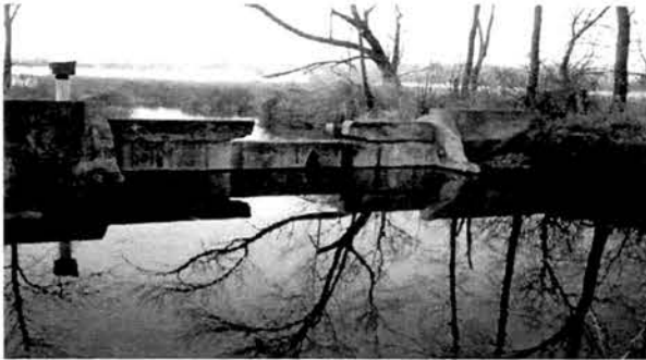
Grove Lake Dam in need of repairs.
