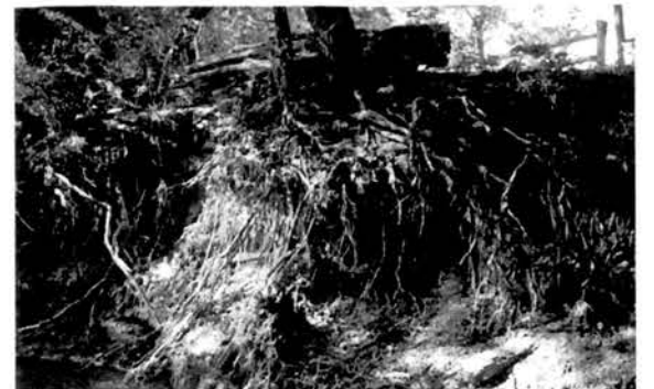
Excessive erosion on CD-32 in 1999 (before).
