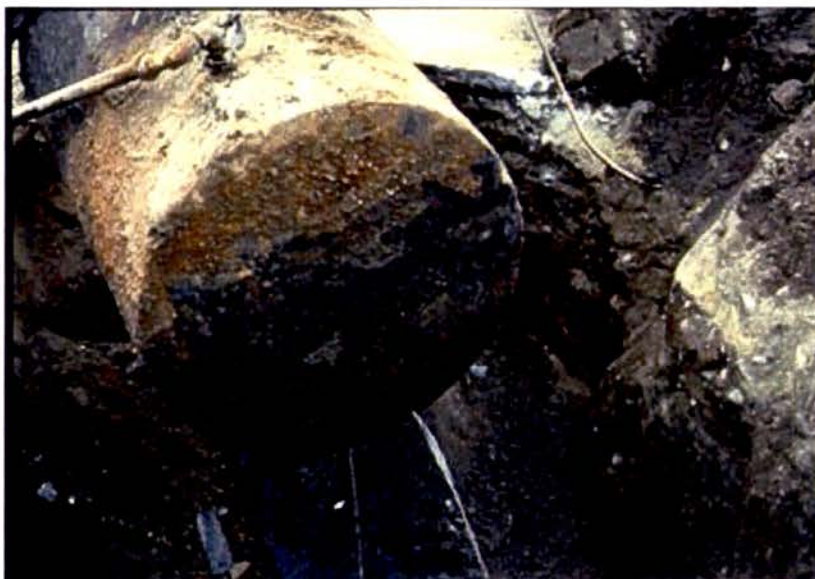
Corroded tanks, improperly filled tanks, overfilled tanks, and poorly monitored tanks lead to petroleum contamination in the soil, ground water, and surface water. New tank installations now include corrosion protection, leak protection, spill protection, and overfill protection.
