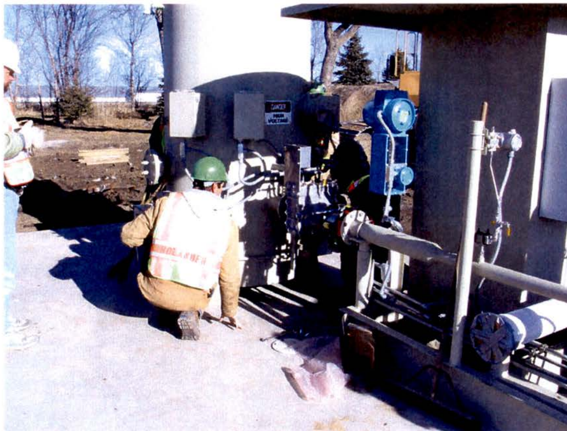
MPCA contractors inspect an enclosed flare system designed to burn off harmful landfill gases.
