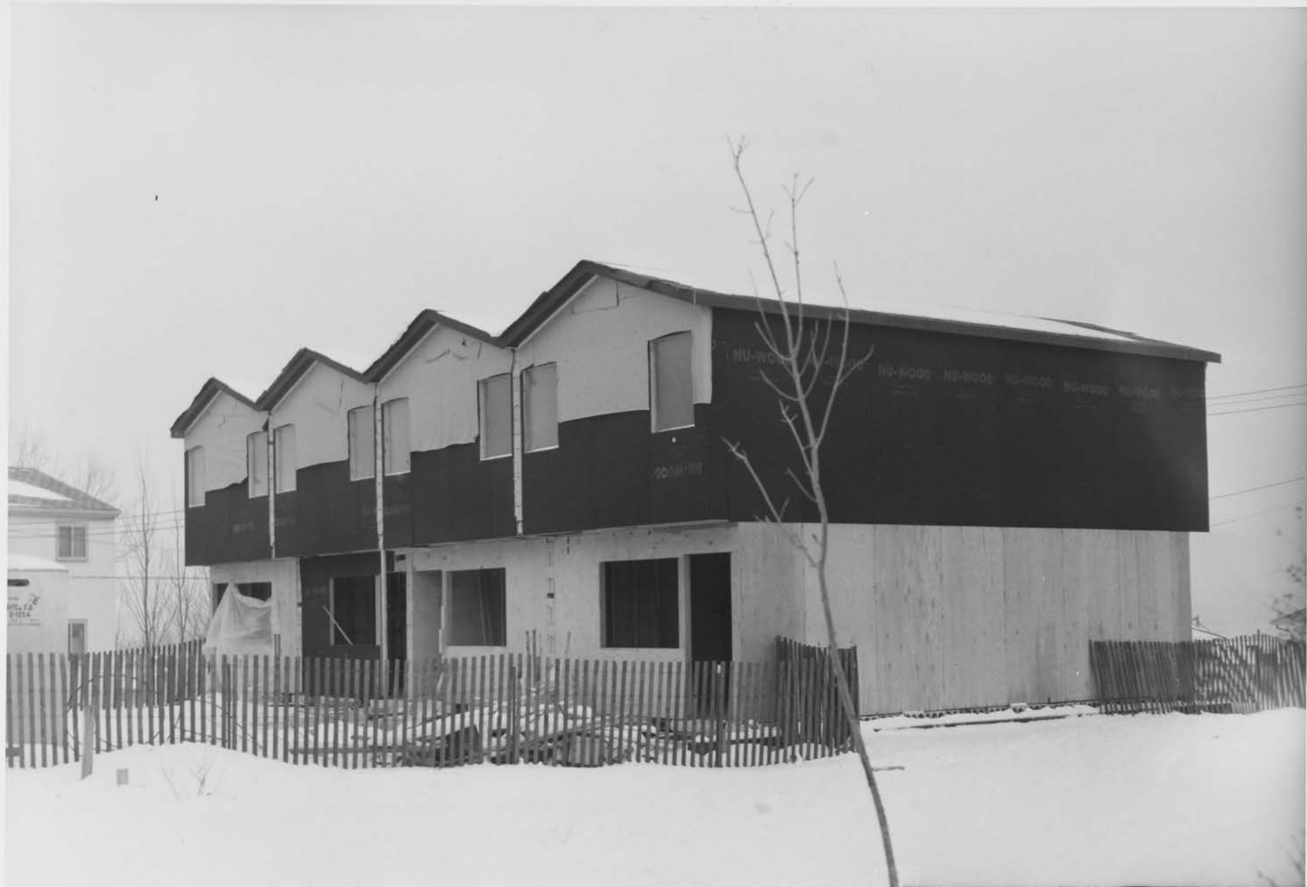
Position H Serial No. 57 Minn. 1-8 Mount Airy Homes Addition. Stage 2 St. Paul, Minn. Date: November 30, 1964 Building No. 2.
