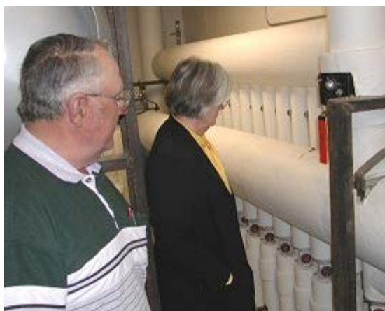
School board chair Wendell Fredin gave Lt. Governor Schunk a tour of the school's state-of-the-art geothermal heating and cooling system
