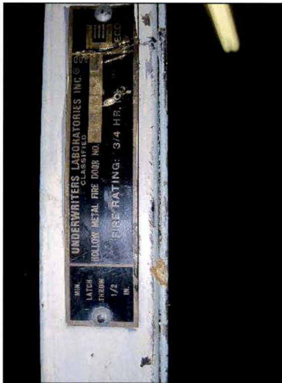
Fire Door Labeled Hollow Metal (No insulation)
