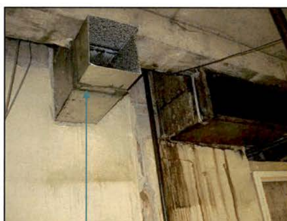
Asbestos Containing Duct Seam Sealant (Sample 21A)
