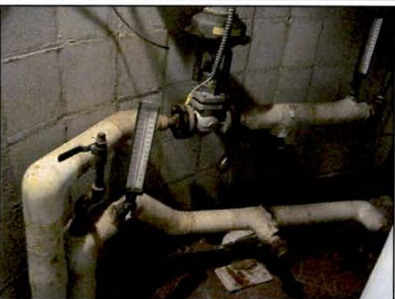
Asbestos Containing Wrap on Pipe Fitting Insulation (Samples 11A-C)
