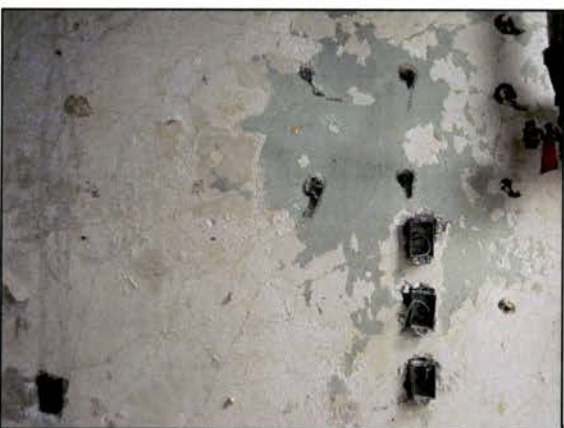
Lead Based Green/Gold Paint on Plaster (PB-18), with Adjacent White Paint (Pb-19)
