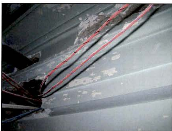
Mezzanine – Lead Based Green Paint on Plaster in the Ceiling Space
