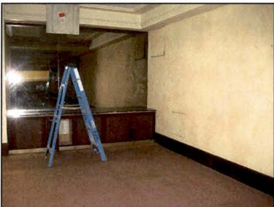
Mezzanine – Mirror and Granite Counter Not Disturbed During Survey (Potential asbestos containing materials behind these items)
