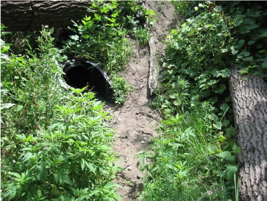
Bottom: Outlet to pond lacking riprap stabilization
