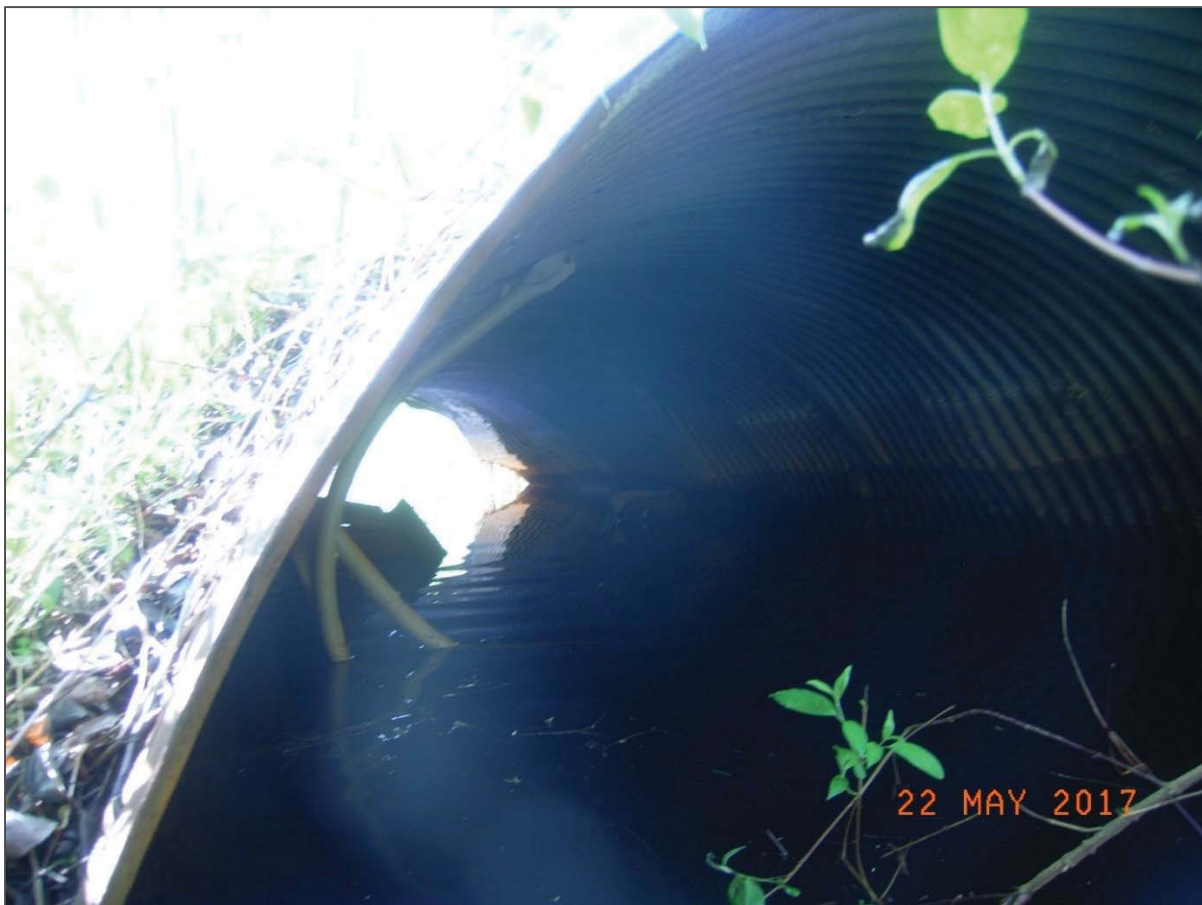
Figure 3: Swing-set frame and other trash found during the May 22 field survey within the 84" CMPA below the field crossing.
