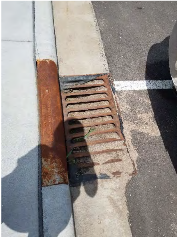
Above photo: Inlet protection in need of maintenance
