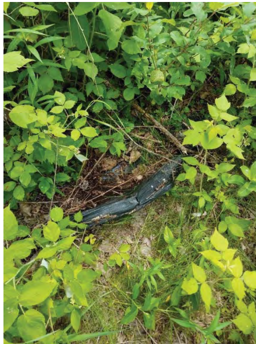
Above photo: Leftover silt fence needing to be removed following final stabilization
