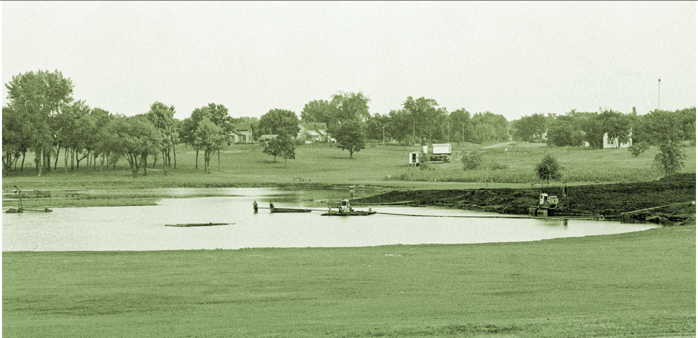
Hard labor by these WPA workers was required to carve the Anoka course and dredge this two-acre lake out of sandy soil and swampland.
