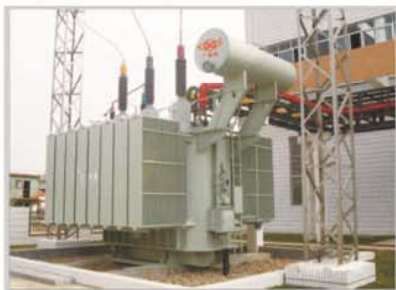
广州凤村变电站110kV主变 Operating in Guangzhou substation 110kV main transformer
