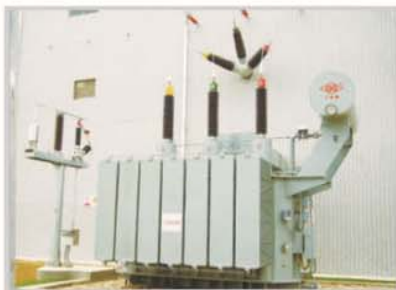
海南感城风电场110kV主变 Operating in Hainan wind power substation 110kV main transformer
