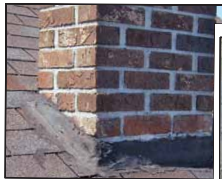
Chimney with cracked and deteriorated flashing
