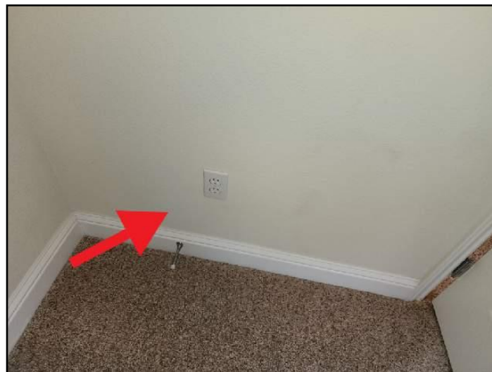
12. Broken Outlet Cover
