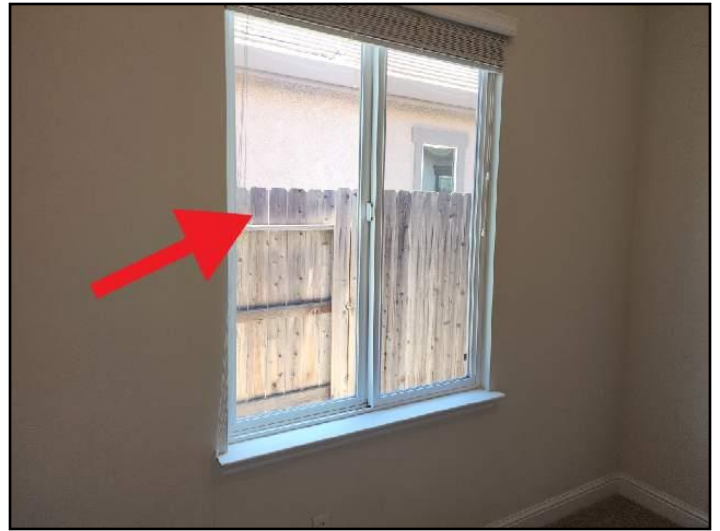
22. Seal Fail(s) Noted
