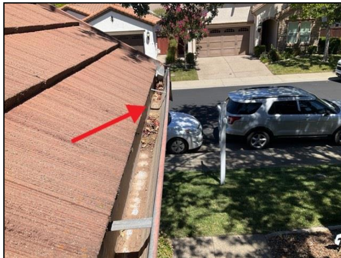
25. Debris/Water Build Up
