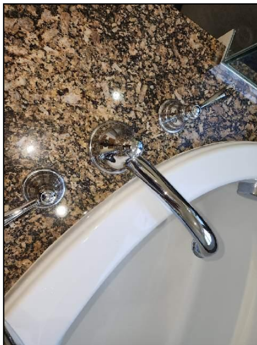
52. Loose Tub Spout
