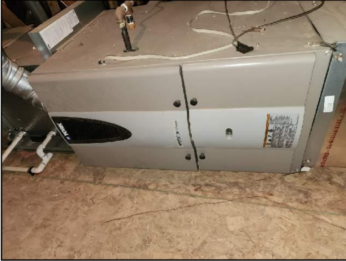
38. Furnace System Info
