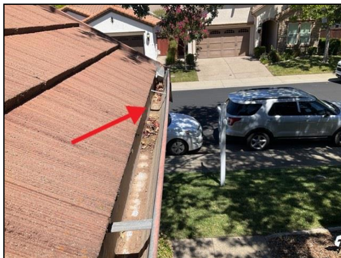
3. Debris/Water Build Up
