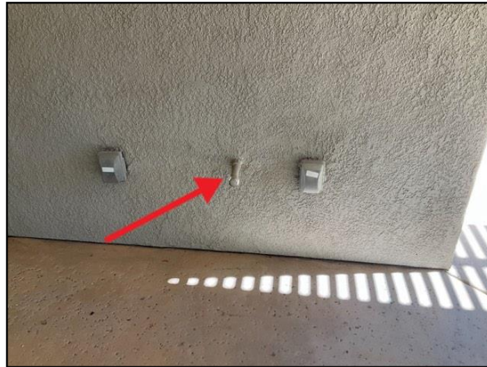
27. Natural Gas or Propane Stub Out
