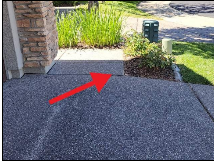
30. Cracks and Lifting at walkway
