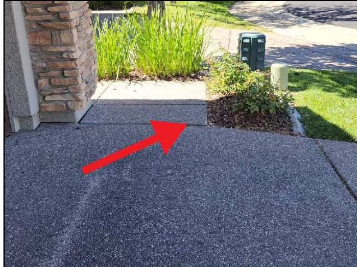
7. Cracks and Lifting at walkway
