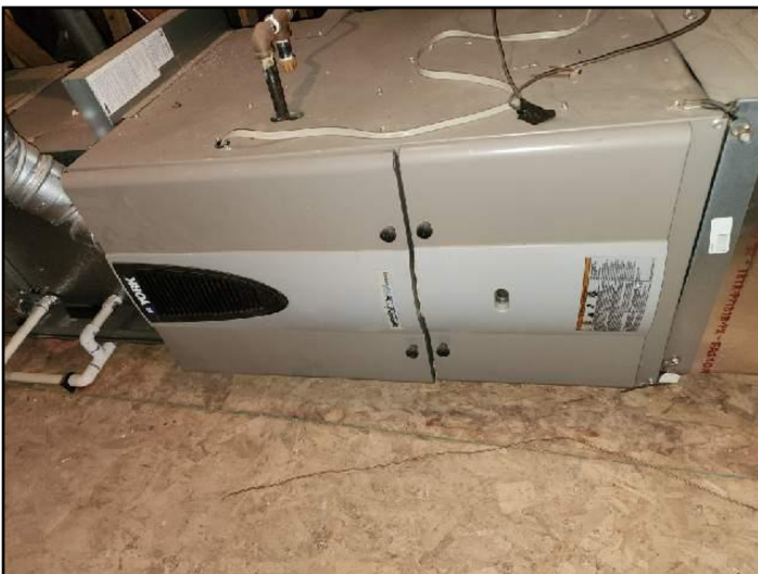
13. Furnace System Info
