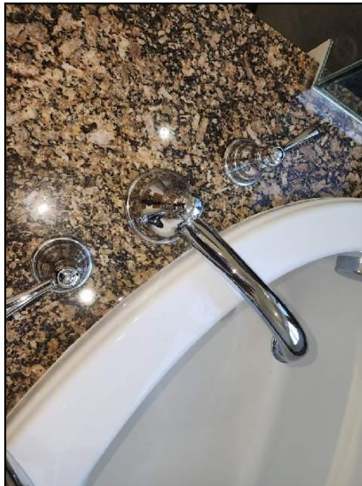
19. Loose Tub Spout
