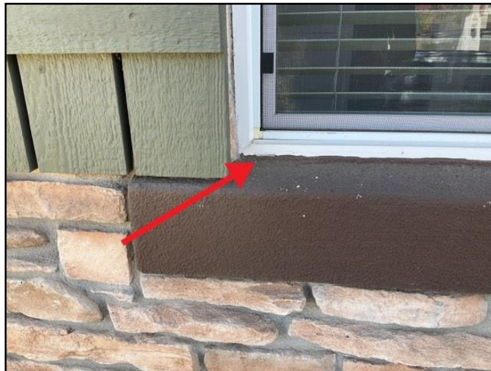
6. Weep Holes Plugged
