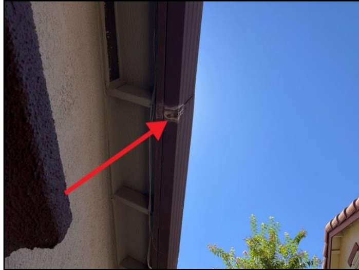
26. Leak at Seams
