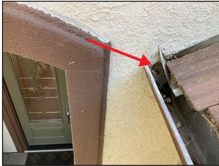
5. Gaps at Siding
