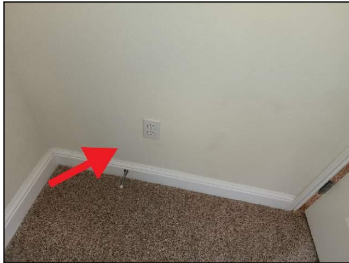
36. Broken Outlet Cover
