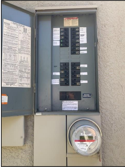
32. Main Panel: Right side of Home
