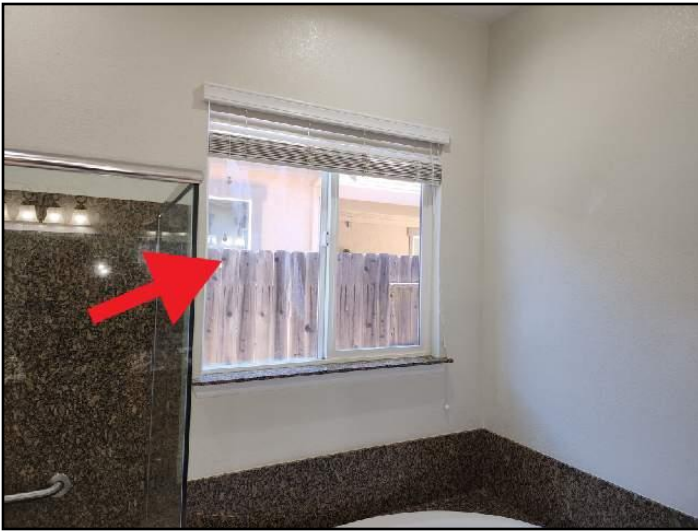
21. Seal Fail(s) Noted
