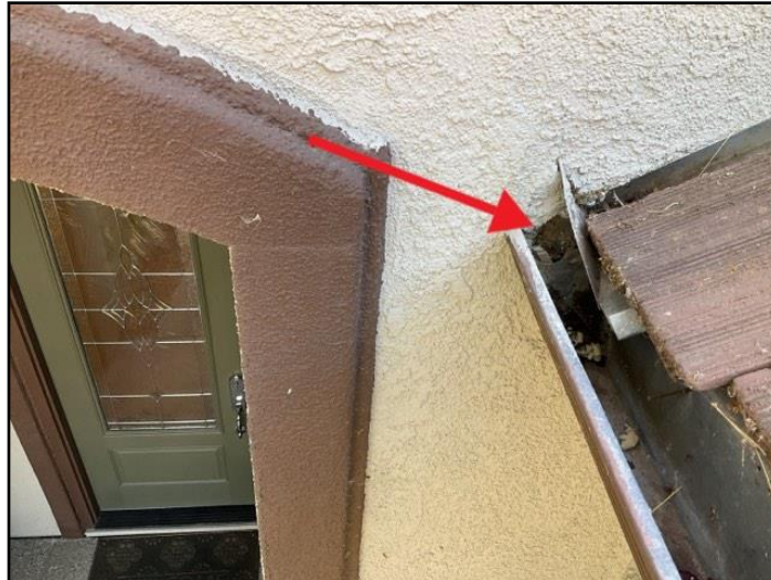
28. Gaps at Siding
