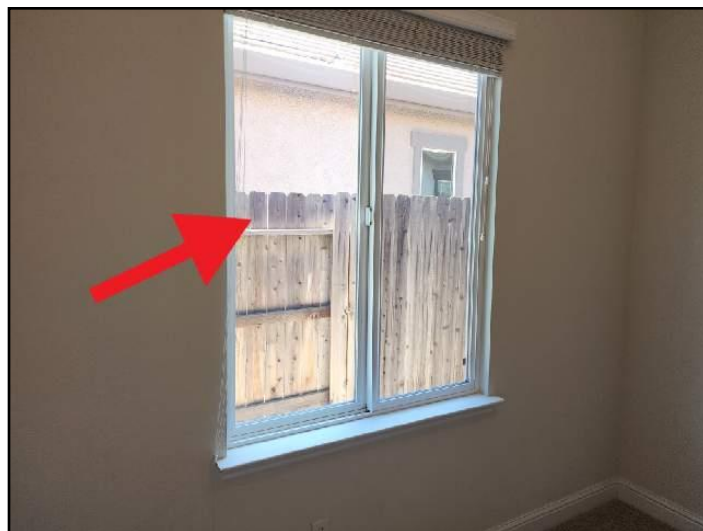
55. Seal Fail(s) Noted
