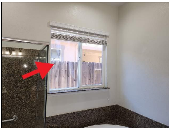
54. Seal Fail(s) Noted
