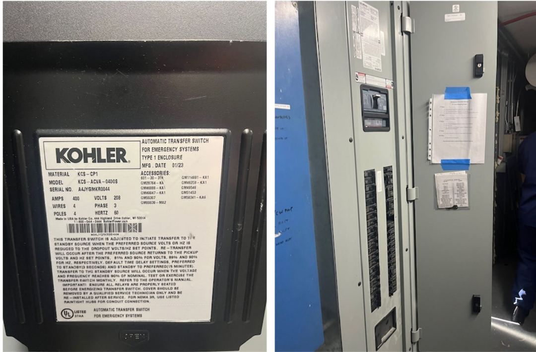
EXISTING ATS (LEFT) AND EXISTING ELECTRICAL PANEL (RIGHT)
