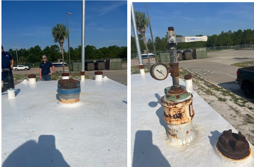
EXISTING RUST TO REMOVE AND TANK TO PAINT.
