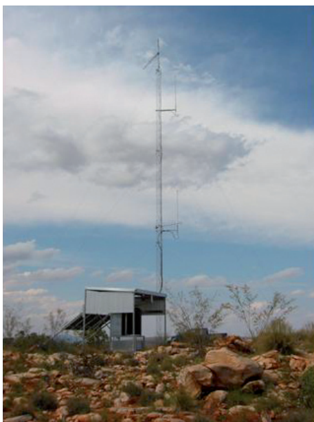
Figure 3.3.3.1: UHF repeater tower at Warakurna settlement
