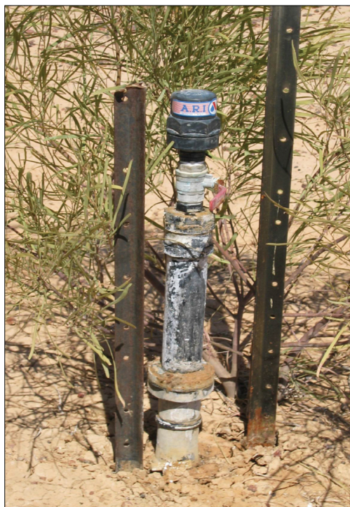
Figure 20: Calcium carbonate deposits on an air valve
