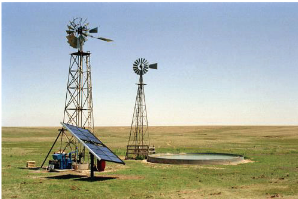
Figure 14: Example of a solar powered pump system
