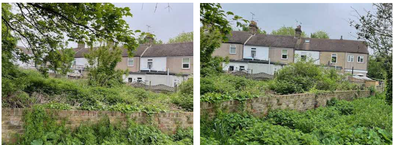
Figure 19. Boundary wall at the southern end of proposed car park plot with Lennard Row Terrace behind.
