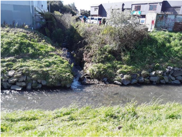
Plate 1: Transect 021/03 – Straightened channel with rock armoring on the true left and some on the true right. Confluence between Porirua mainstem and Mitchell Stream.
