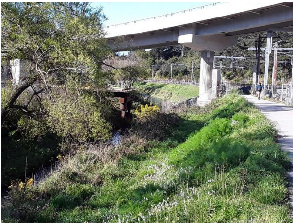
Plate 3: Transect 021/05 – Bank stabilisation structures present downstream. Stream in close vicinity to walkway.
