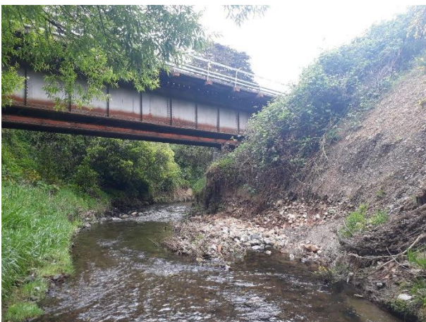
Plate 19: Transect 024/04 – Erosion of streambank. Blackberry present.
