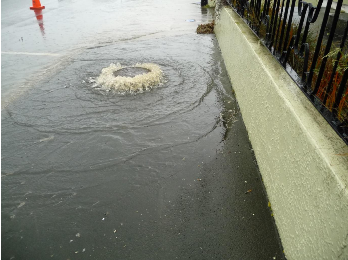
Surcharging Manhole on Mana Esplanade in Heavy Rain
