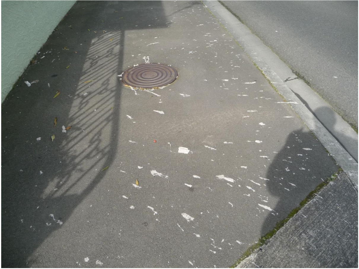
Toilet Paper from Manhole on Mana Esplanade after Heavy Rain
