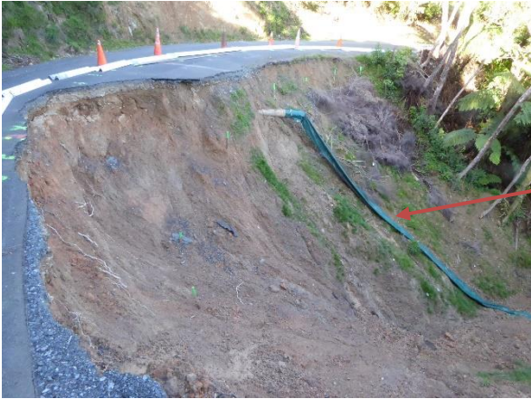
Culvert discharge control
