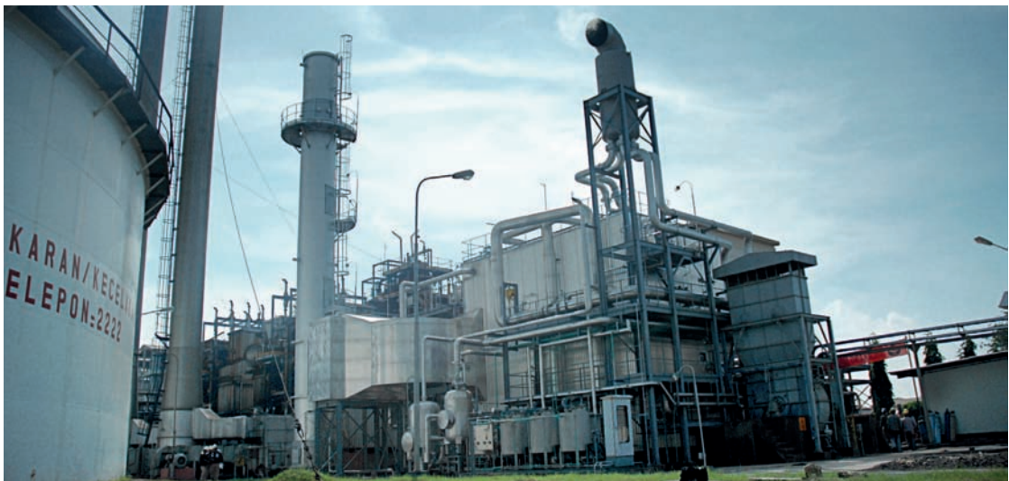
Gas Turbine Generator
