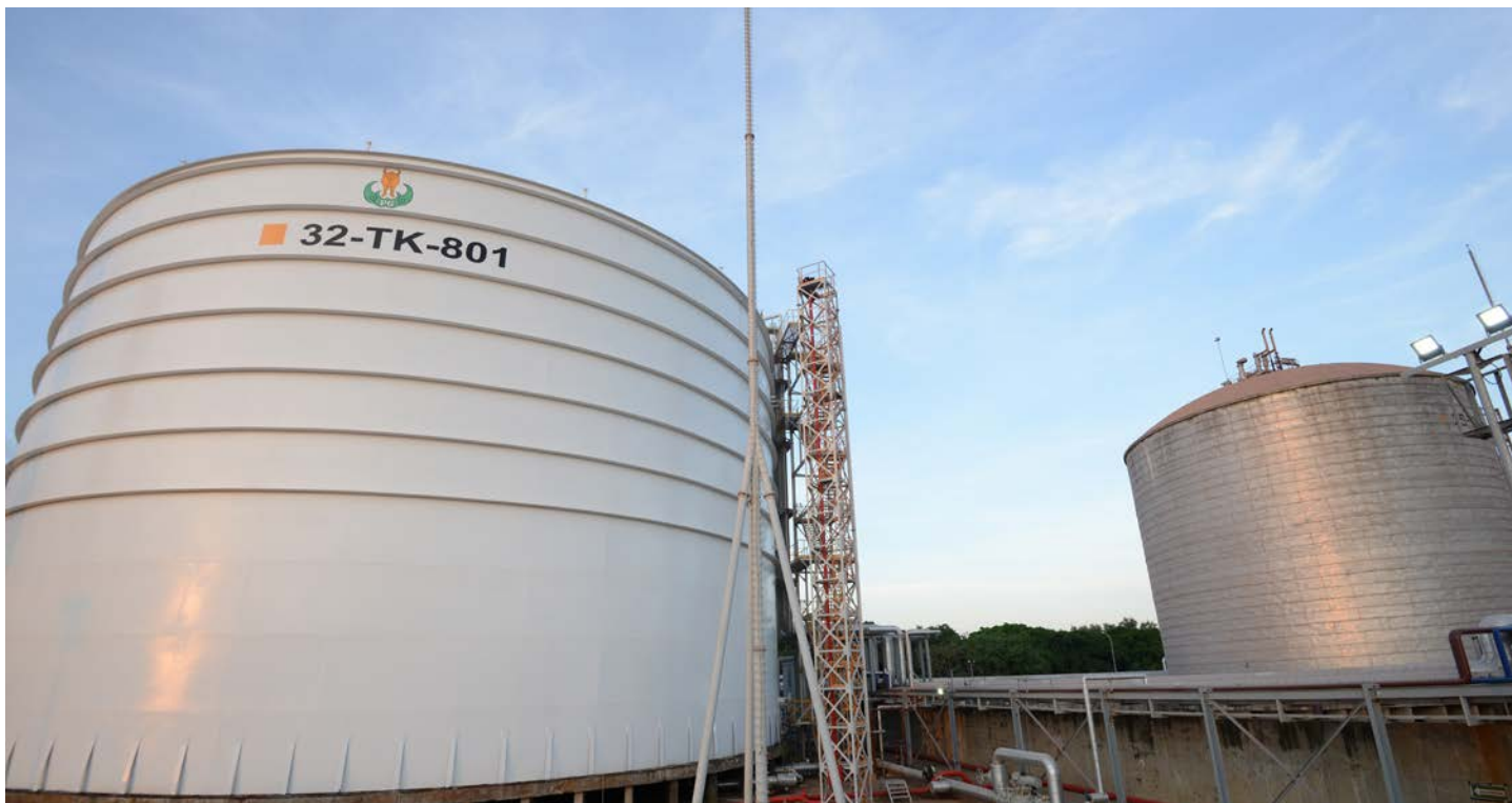
Pabrik Revamping PA akan meningkatkan kapasitas produksi Asam Fosfat PG PA Revamping Plant will increase production capacity of PG Phosphoric Acid
