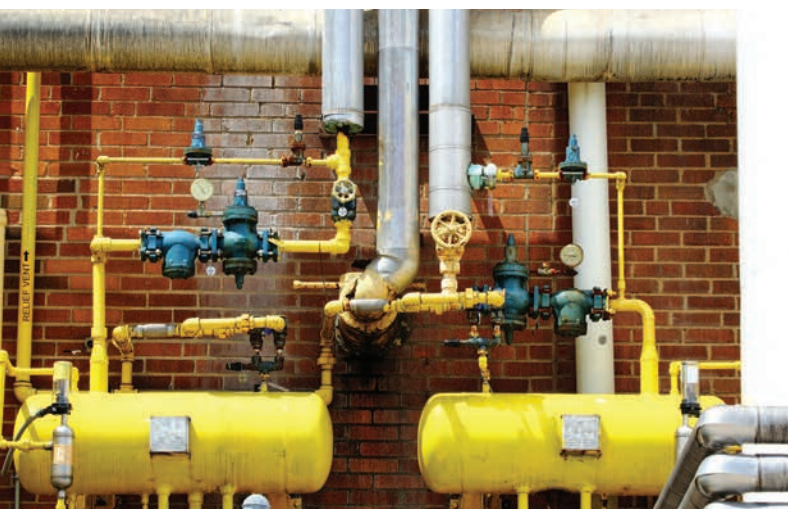
Above: Ammonia refrigeration tanks.
