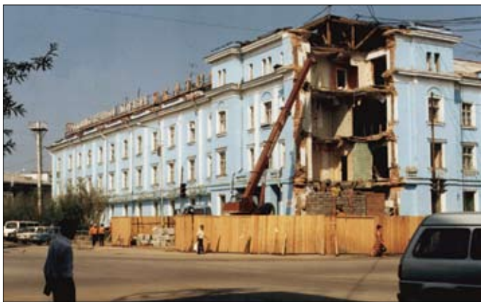
Fig. 12. Collapse of a corner of a building located in the centre of Yakutsk, 1999 (Photo by M. P. Grigoryev) (Alekseeva et al., 2007).
