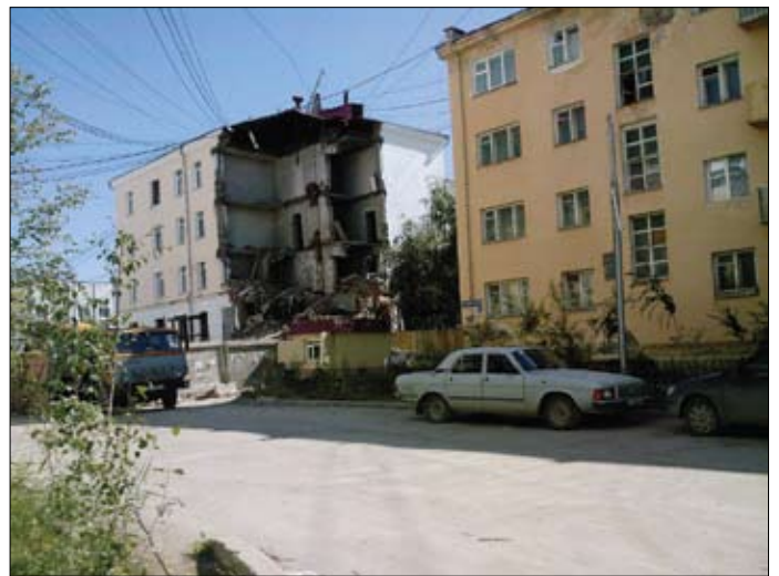
Fig. 13. Collapse of a part of the building belonging to the Administration for Geological Surveys in Yakutsk, 2009 (Photo by M. P. Grigoryev)
