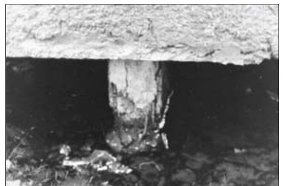
Fig. 15. A residential house in an emergency state, Dudinka. An inspection revealed that the wall subsidence has been caused by erosion, destroying reinforced steel piles in the basement. Photo by V.Grebenets.
