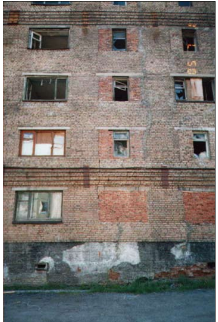
Fig. 9. On the top, an unsafe and irreparable house. Residents were moved to other residences. Vargashor Street 14, Vorkuta
