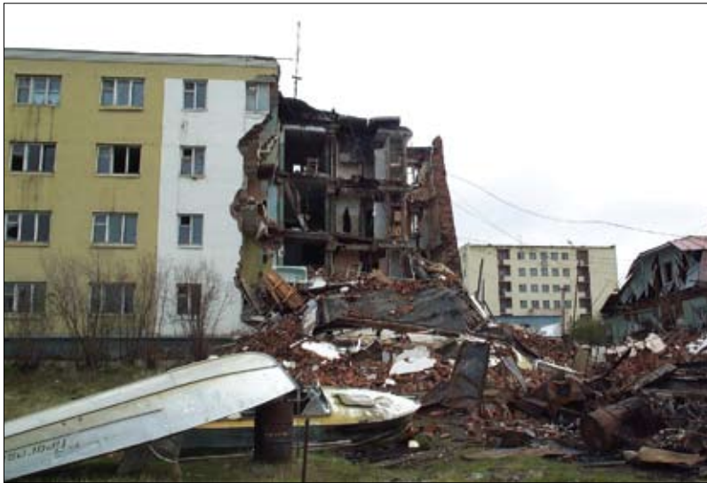
Fig. 14. A building section collapsed due to weakened basement, Chersky village. (Photo by V. E. Romanovsky)
