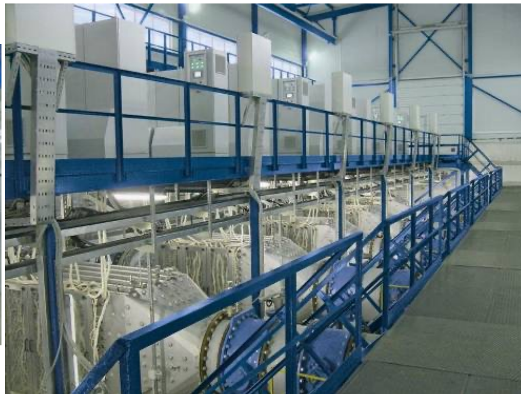
North WTP. 18 units
