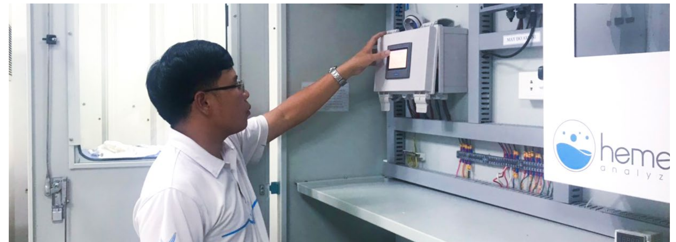
Photo of Automatic WW monitoring system
