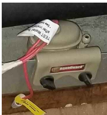
Drain Pan Float Switch
