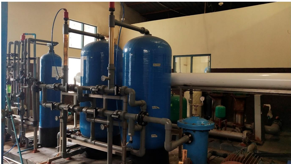
Figure 22: existing RO plant
