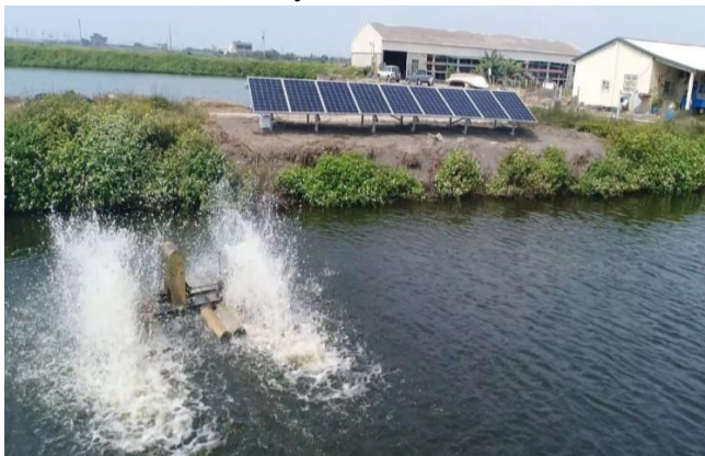
Paddle Aerator System
