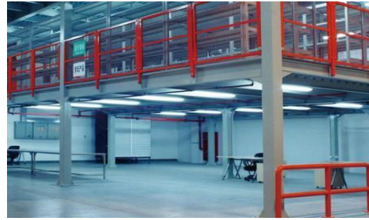
Heavy Duty Warehouse Multi-tier Steel platform
