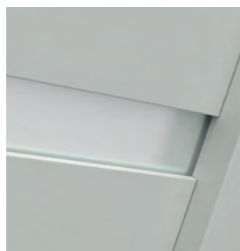
glazing of G.4 model - glass panel recessed in comparison to the surface of a door panel
