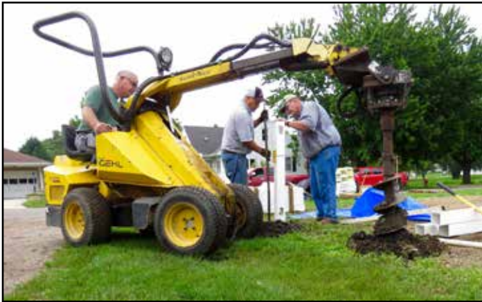
Mark LeGare and Joe Maidl straightened and tamped the first post for the kiddie park fence while Dean Koppelman of Rohlfin's drilled the second hole. The posthole digger made the work faster and much easier!
