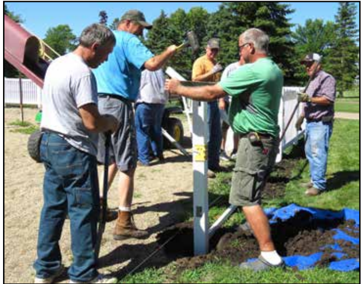
After the holes were dug, the posts were set in, pounded down to the right height, then tamped and filled with dirt and Sakrete. Workers are, from left: Steve Sjostrom, Dale Bjorklund, Joe Maidl (back), Mark Dick, Dwight DeBoer (hidden), Dean Koppelman from Rohlfin's, and Mark LeGare. Others helping with the project were Arden DeBoer, Andrew Maidl and Ruth Klossner.
