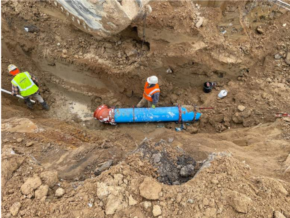
Photo #1: Installing 45-degree fitting at the intersection of Aztec Road and Highway 10 - Jan 22, 2024, 2:26 PM
