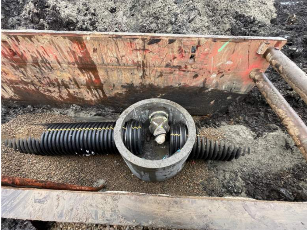
Photo #6: BP MH-9 in place with 30" gravity flow pipes in either side - Jan 25, 2024, 2:50 PM
