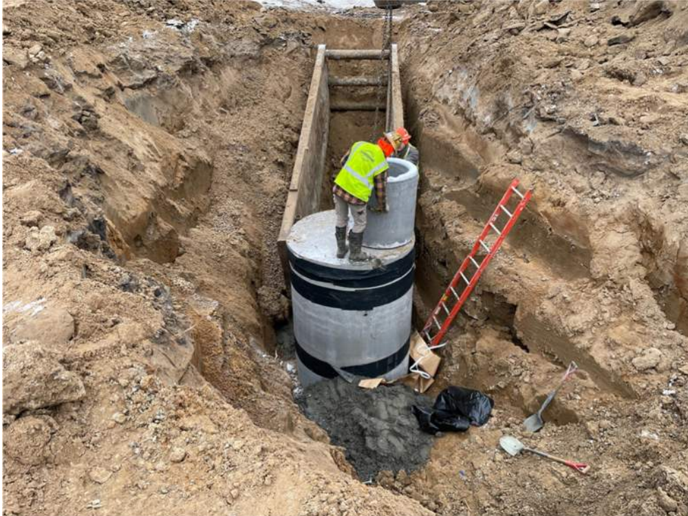
Photo #2: Installing the small riser section on top of the manhole - Jan 23, 2024, 8:58 AM
