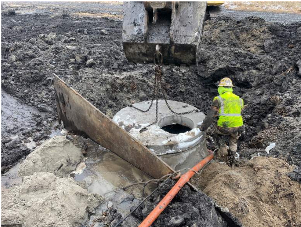
Photo #7: Putting the top slab on a manhole in the swamp - Jan 25, 2024, 2:55 PM
