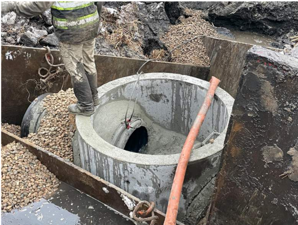
Photo #5: Concreting the pipes in and around the entire manhole and base slab - Jan 24, 2024, 3:59 PM
