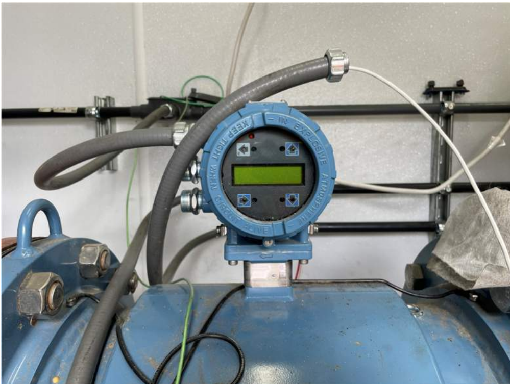
Photo #4: Magnetic flow meter situated and being hooked up - Jun 19, 2024, 9:39 AM
