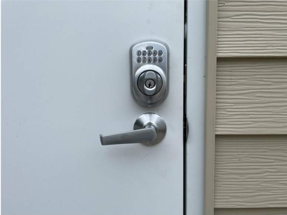
Photo #3: Door handle and lock installed on pump house service door - Jun 17, 2024, 3:45 PM
