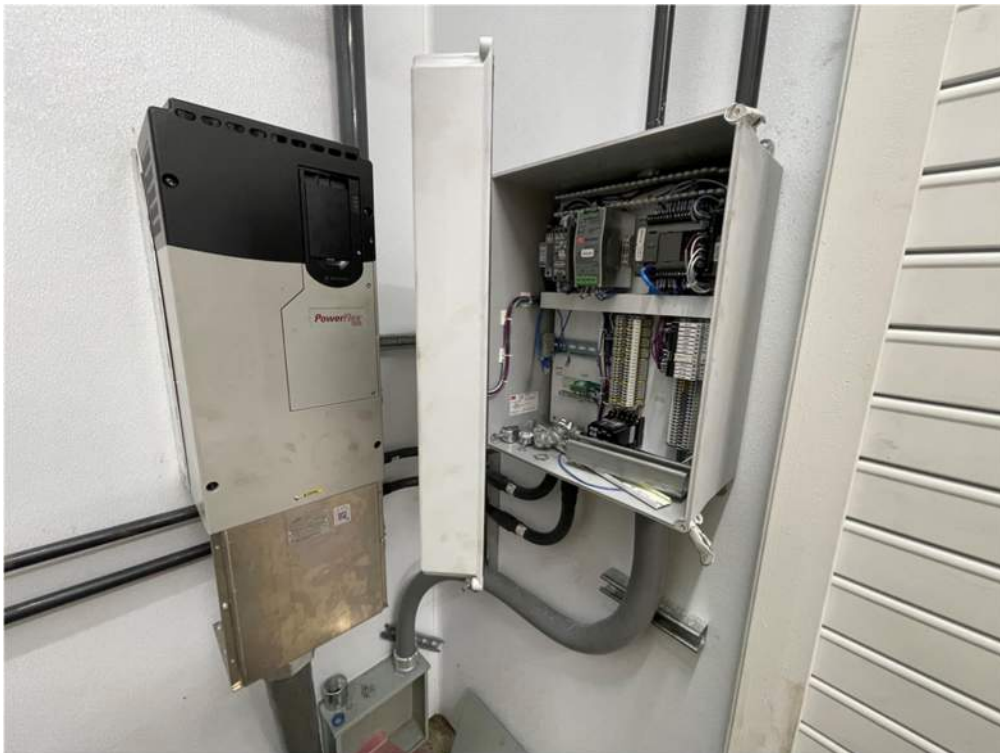
Photo #2: Electrical work on the North wall of the pump house - Jun 17, 2024, 3:44 PM
