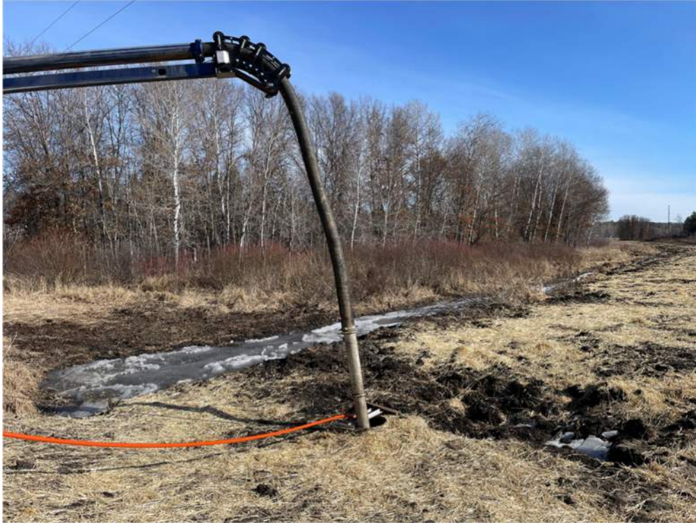
Photo #2: Jetting and vacuuming the water and sediment from inside the pipe into the swamp and along Atlantic Road - Feb 26, 2024, 10:37 AM
