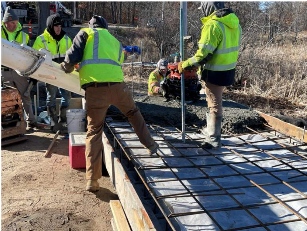
Photo #5: Signature M Concrete is pouring the concrete for the floor of the pump station - Feb 29, 2024, 10:16 AM
