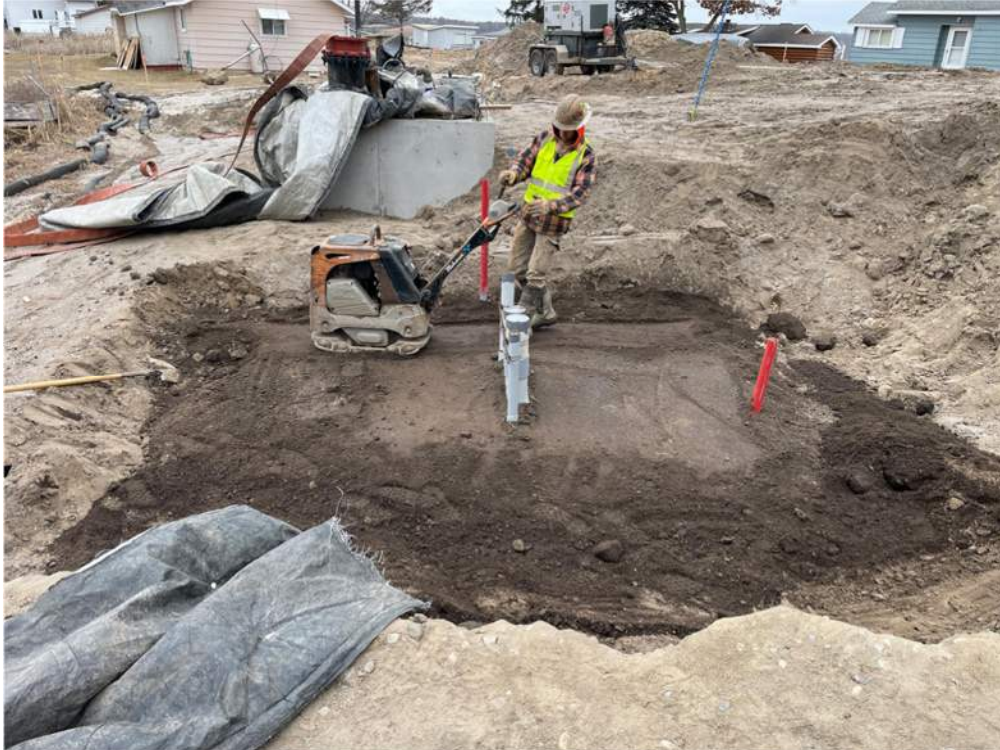
Photo #4: Compacting soil where the transformer pad is to be poured near the pump station - Feb 27, 2024, 1:25 PM
