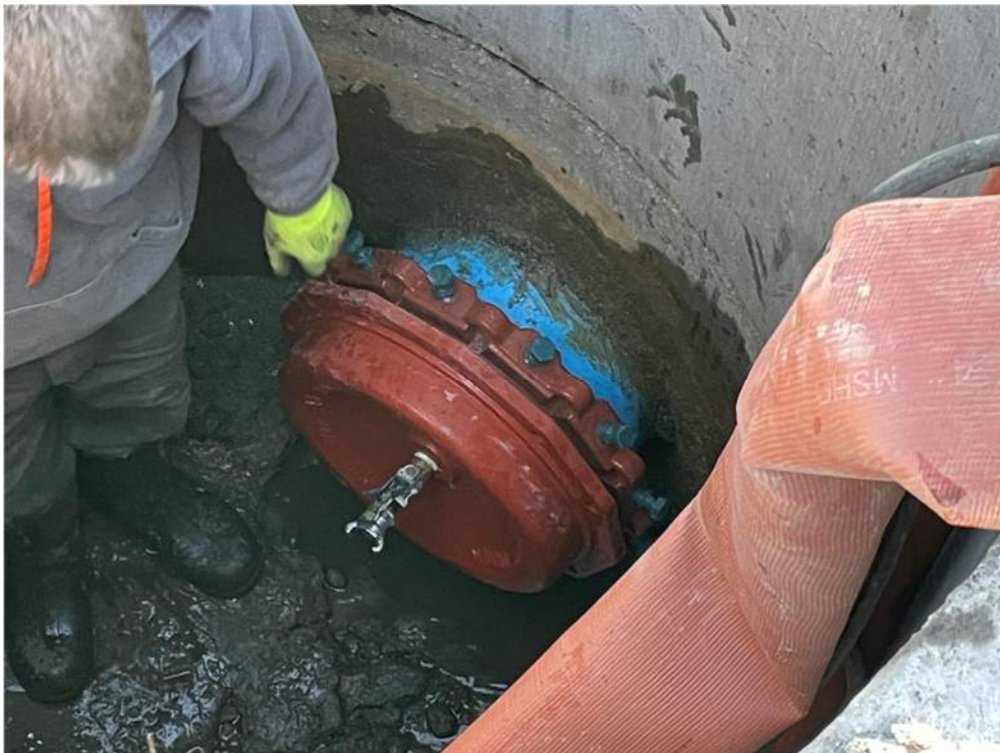
Photo #7: Landwehr installed a temporary cap on the end of the force main to prepare for pressure testing the pipe - Mar 1, 2024, 7:53 AM
