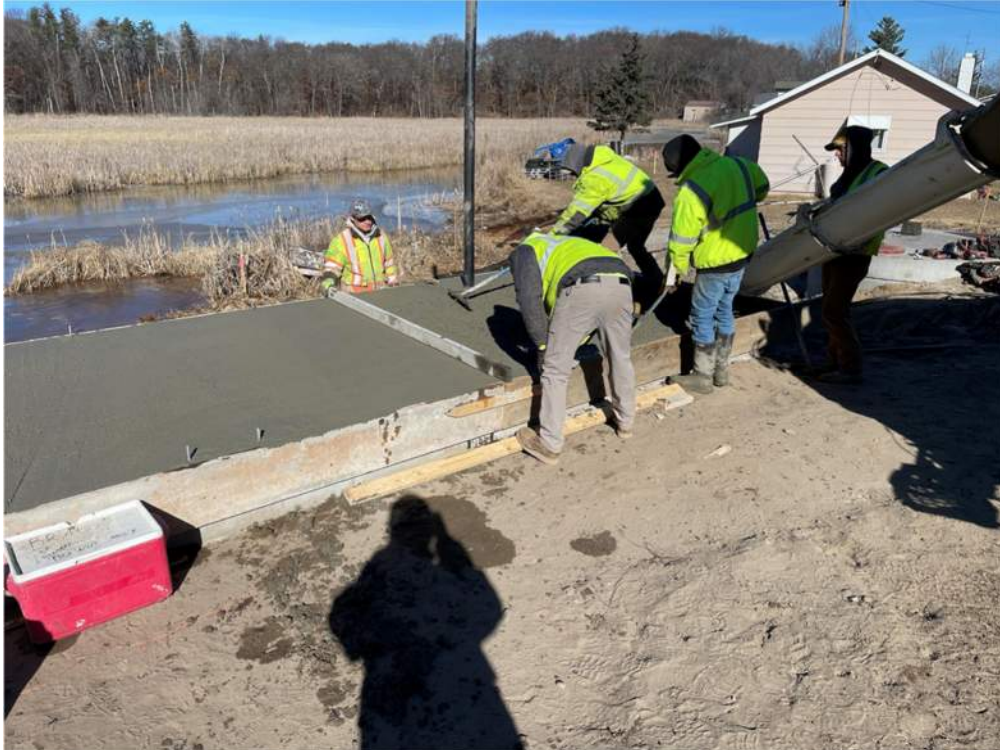
Photo #6: Signature M Concrete is vibrating and leveling the concrete for the pump house floor slab - Feb 29, 2024, 10:25 AM
