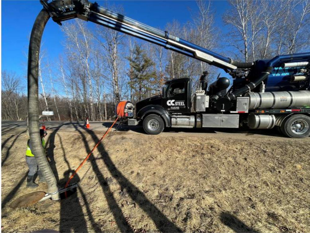
Photo #8: CC Steel is continuing to jet and vacuum any debris left in the gravity flow pipe along Pulaski Road - Mar 1, 2024, 9:22 AM
