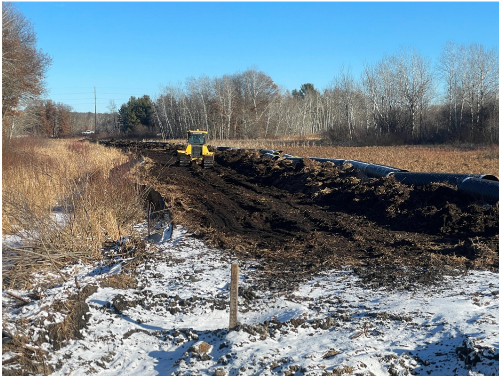
Photo #5: Stripping topsoil prior to pipe installation west of Hwy 10- Dec 12, 2023, 2:13 PM
