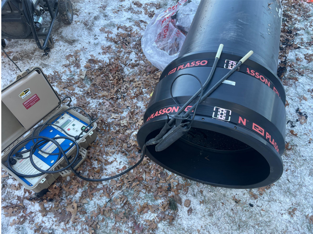
Photo #4: Fusing coupling to 24" gravity flow pipe from lake inlet - Dec 12, 2023, 11:19 AM
