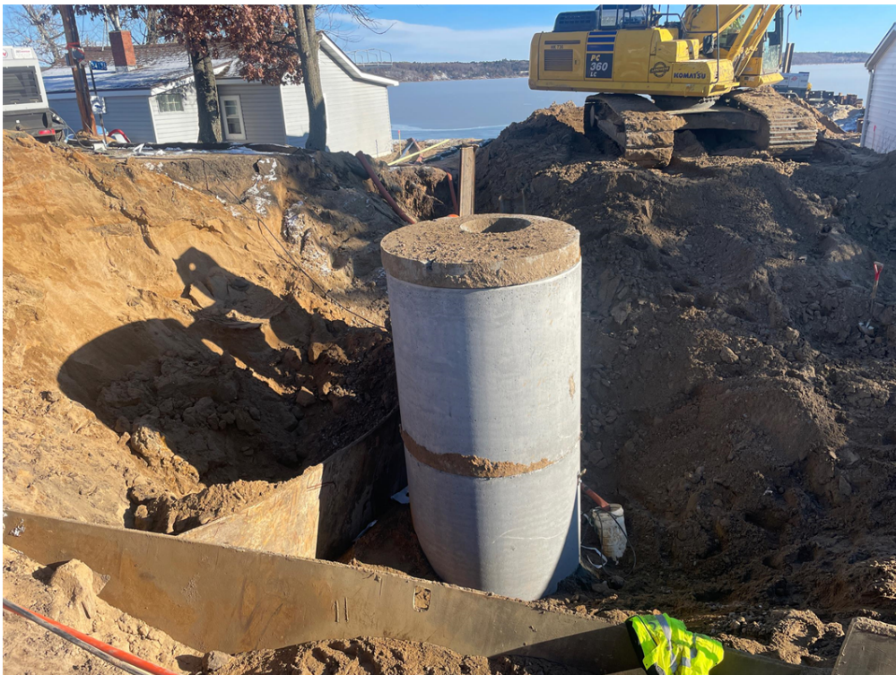
Photo #3: Cover installed on top of manhole in Aztec Rd - Dec 12, 2023, 11:04 AM
