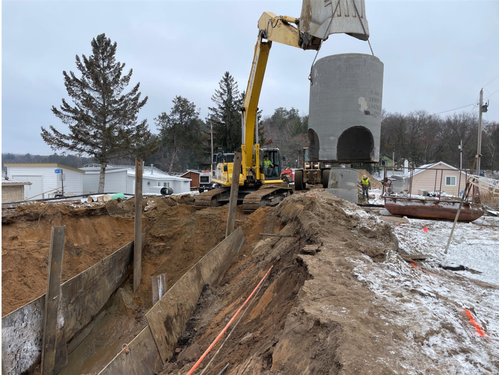
Photo #2: Lowering 8' manhole riser section into trench for installation in Aztec Rd- Dec 11, 2023, 1:19 PM
