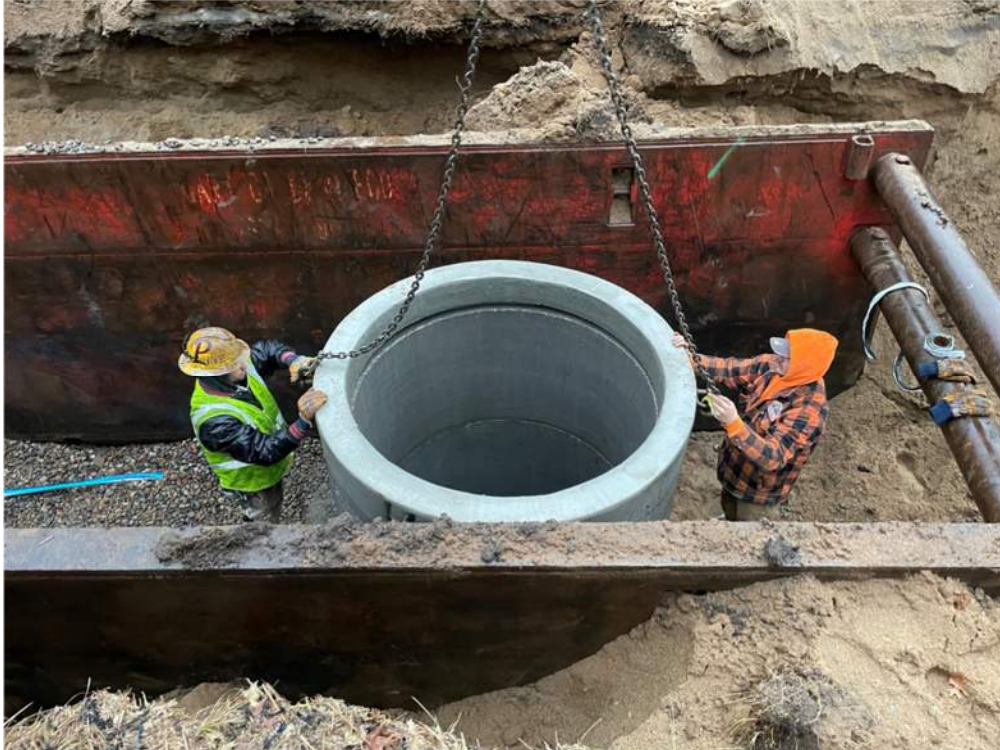
Photo #6: Installing riser sections on top of FM MH-4, Along Aztec Road - Feb 8, 2024, 7:56 AM
