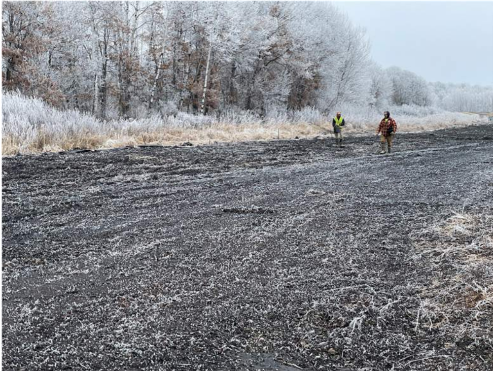
Photo #1: Hand seeding the backfill in the swamp, Near Atlantic Road - Feb 5, 2024, 10:31 AM
