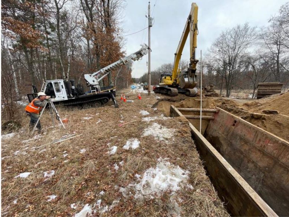
Photo #4: Checking the elevation of the force main pipe, Near Station 170+00 alongside Aztec Road - Feb 7, 2024, 2:20 PM
