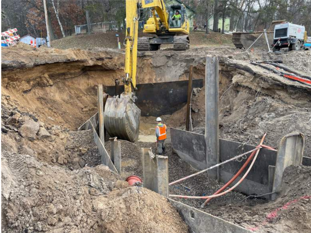
Photo #2: Excavating through Aztec Road to install the road crossing for the force main pipe - Feb 6, 2024, 8:55 AM
