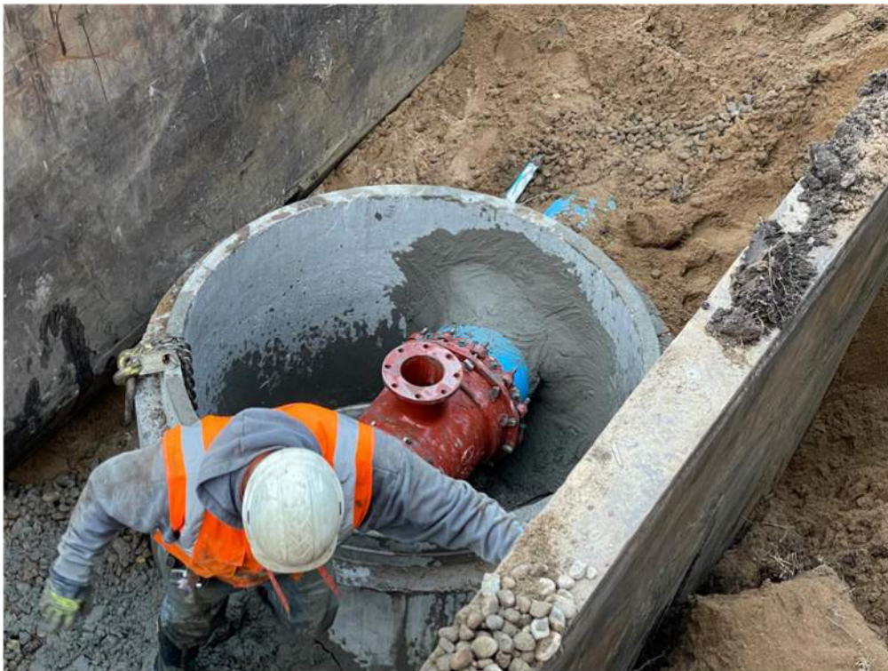
Photo #5: Concreting the hole where the pipe was installed through, FM MH-4 alongside Aztec Road - Feb 7, 2024, 5:10 PM
