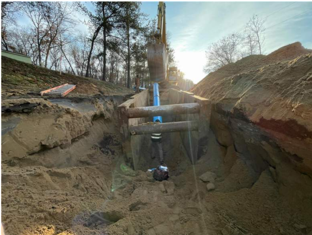
Photo #3: Lowering force main pipe into trench, Along Aztec Road near Station 172+50 - Feb 6, 2024, 4:13 PM
