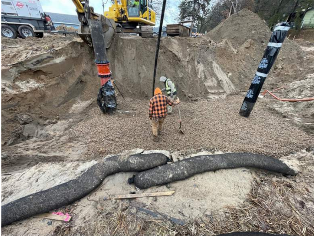
Photo #8: Excavating soil in preparation for the footing to be poured for the pump station - Feb 8, 2024, 2:03 PM
