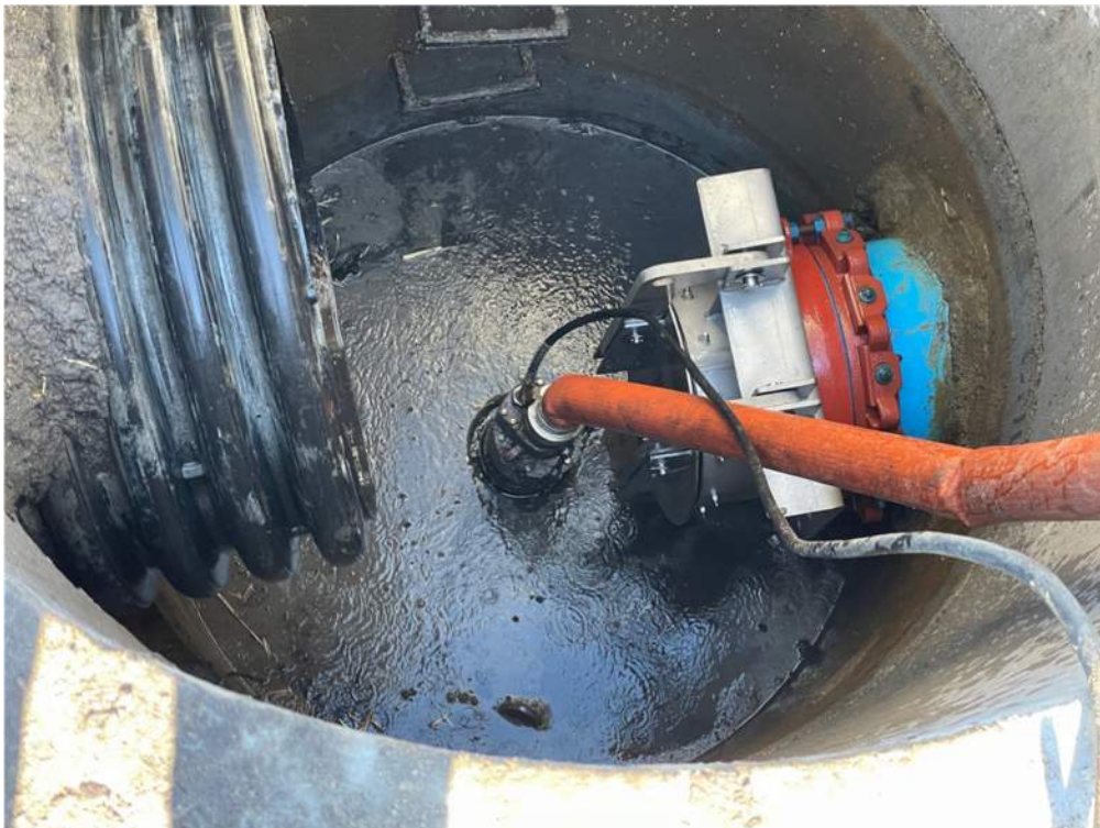
Photo #7: Force main outlet structure has been cleaned out and the flap gate has been installed on the end of the force main pipe - Mar 7, 2024, 11:35 AM
