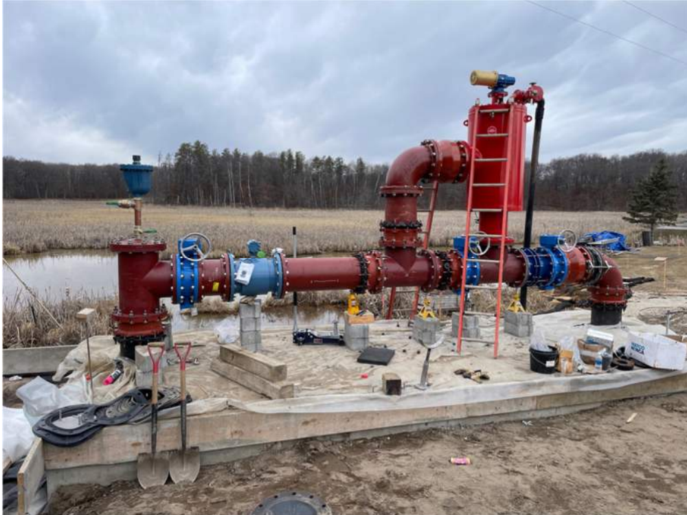
Photo #4: Fittings, pipes, and filter bolted in place in pump house - Mar 6, 2024, 2:56 PM
