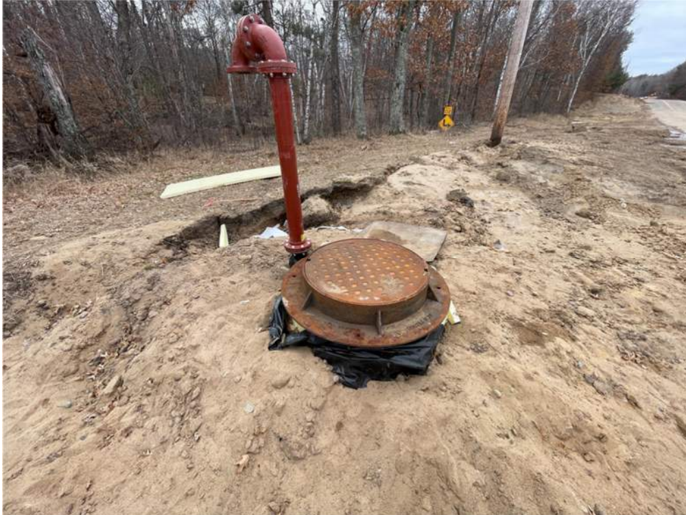
Photo #8: Rings and casting set on one of the AV/AR manholes - Mar 8, 2024, 12:01 PM
