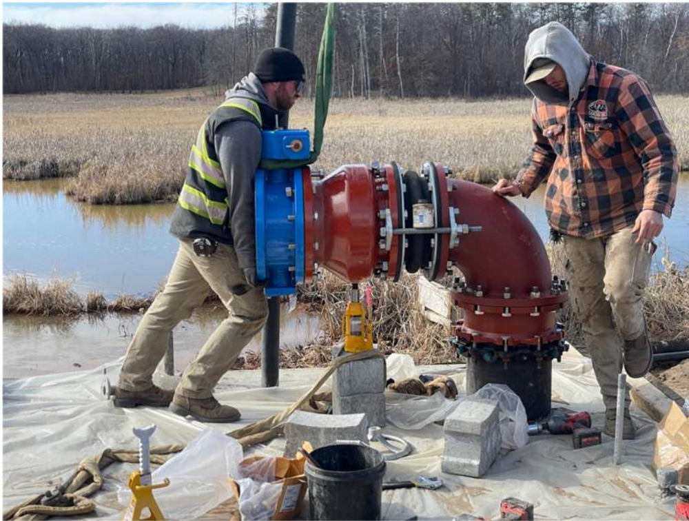
Photo #1: Installing a butterfly valve next in the force main line - Mar 4, 2024, 2:54 PM
