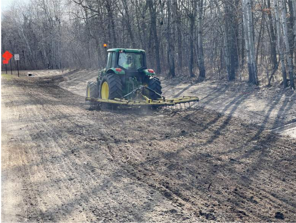
Photo #1: Dragging the surface topsoil to prepare it for seeding, along Aztec Road - Apr 15, 2024, 10:19 AM
