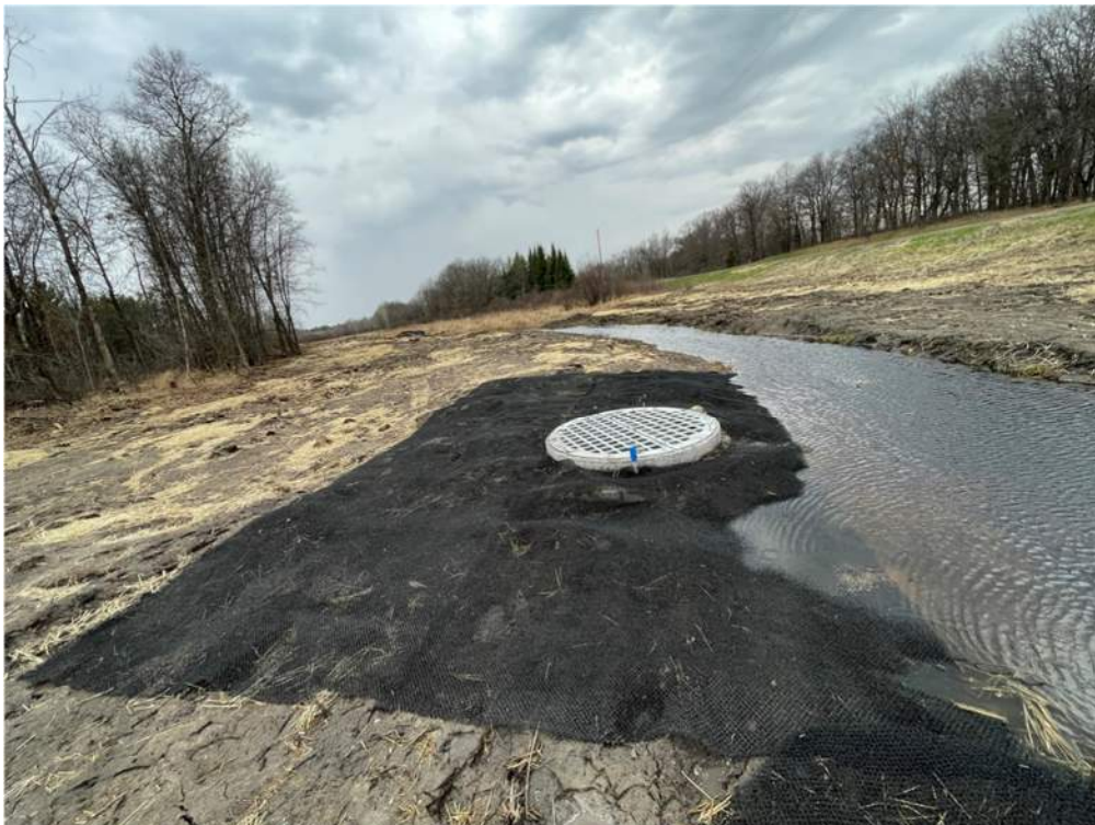
Photo #7: Turf reinforcement mat installed around the force main outlet structure - Apr 16, 2024, 8:38 AM
