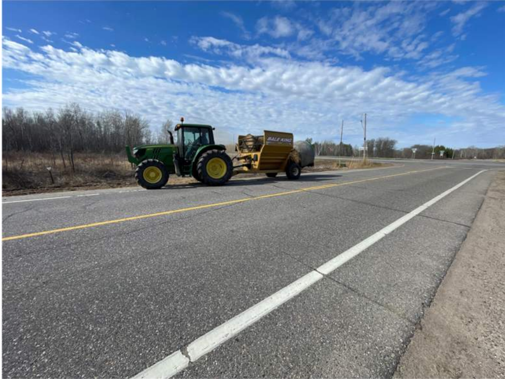
Photo #2: Chopping up bales to cover the seeded areas, near station 104+40 - Apr 15, 2024, 10:23 AM
