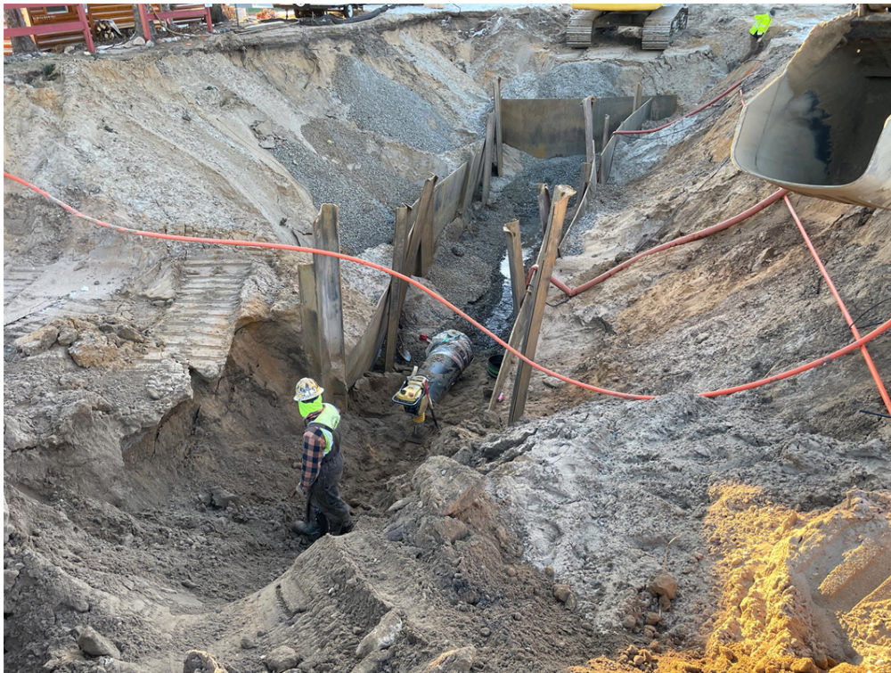
Photo #1: Preparing the trench for the next length of gravity flow pipe - Dec 18, 2023, 8:46 AM
