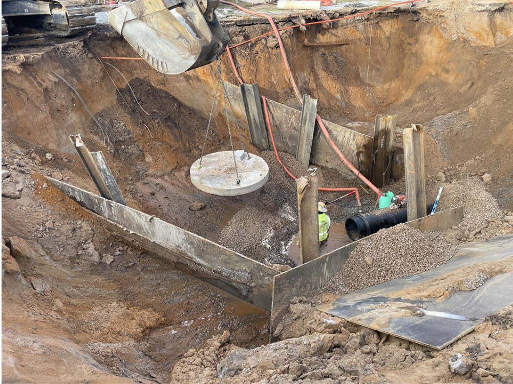
Photo #2: Lowering base slab for manhole into trench to be set - Dec 19, 2023, 10:14 AM
