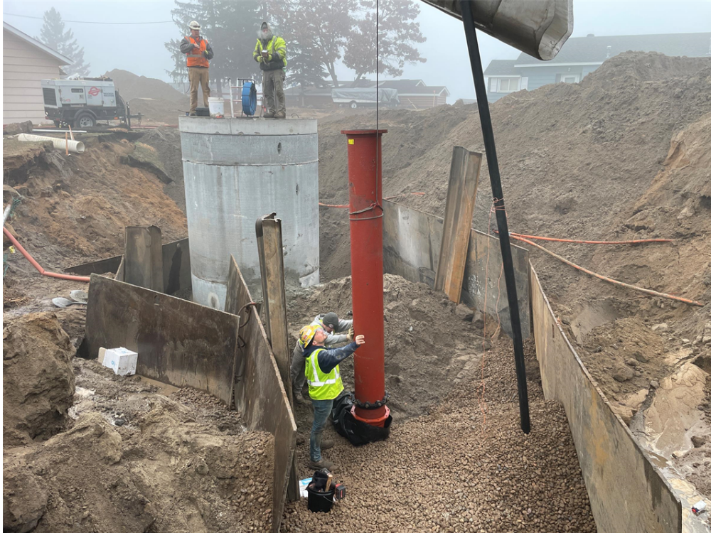
Photo #8: Installing pipe going from wet well to pump station - Dec 22, 2023, 9:03 AM
