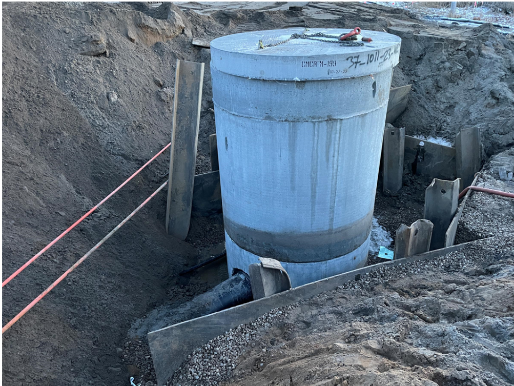
Photo #5: Wet well structure in place with top slab added - Dec 20, 2023, 4:47 PM
