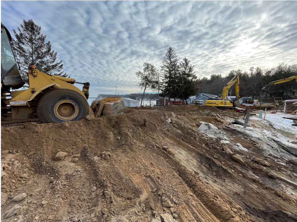
Photo #3: Backfilling over the top of the gravity flow pipe and backwash pipe on Aztec Road - Dec 19, 2023, 11:00 AM
