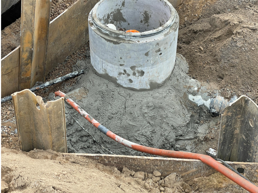
Photo #6: Concreting in pipes going into and out of manhole structure in Aztec Road - Dec 21, 2023, 10:44 AM
