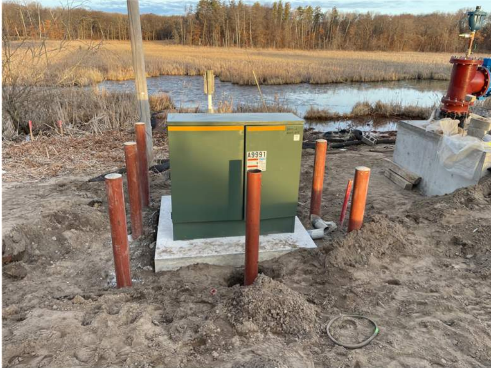
Photo #1: Transformer set on concrete pad - Mar 14, 2024, 8:05 AM
