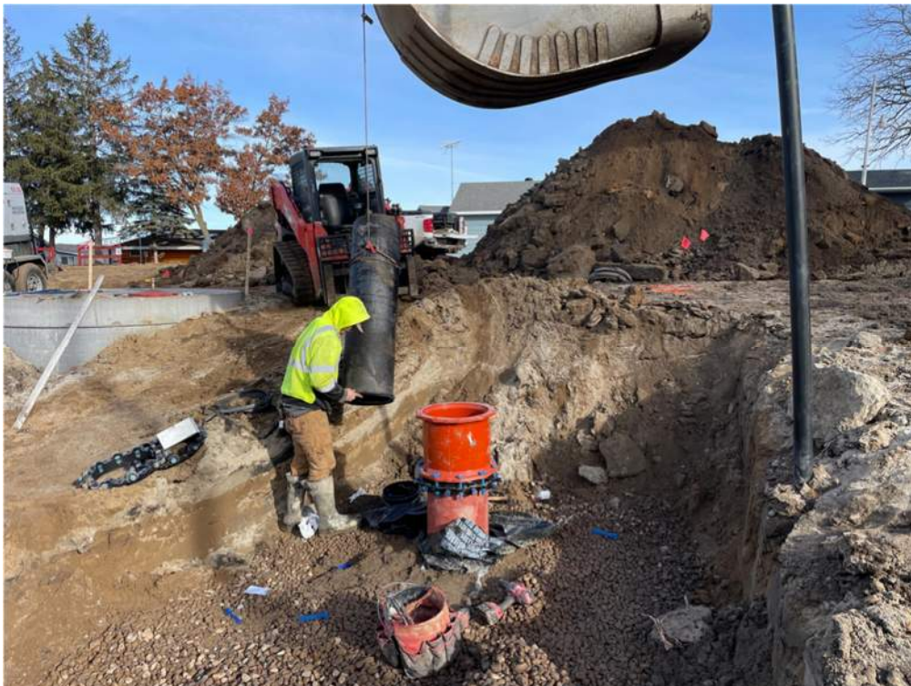
Photo #7: Installing riser pipe section for incoming 14" pipe for the pump station - Feb 1, 2024, 2:12 PM
