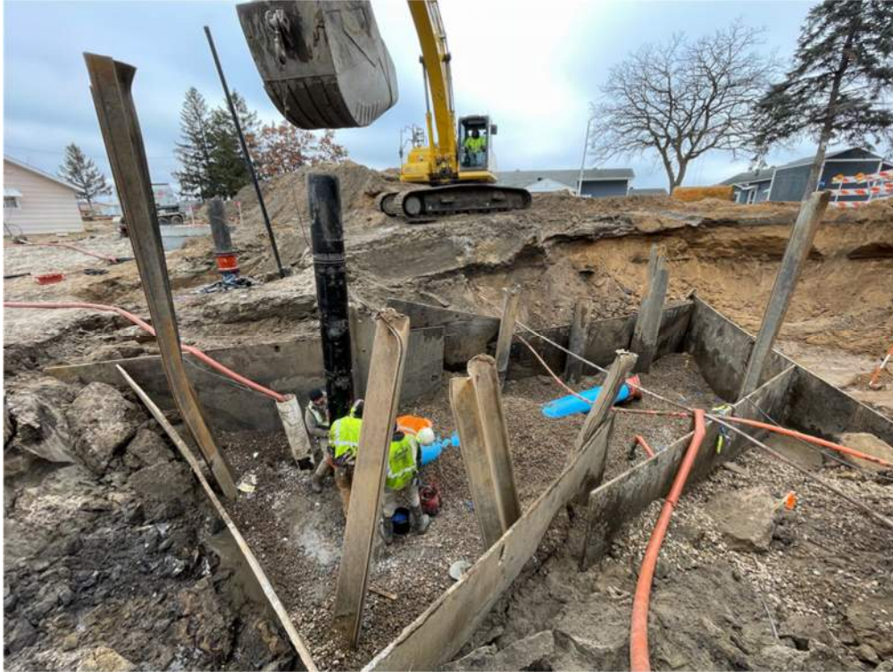
Photo #8: Installing riser pipe to serve as the outgoing pipe in the pump station - Feb 2, 2024, 12:56 PM
