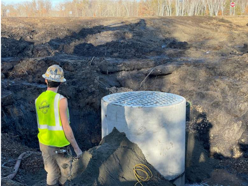
Photo #6: Metal grate for the force main outlet structure - Jan 31, 2024, 3:38 PM
