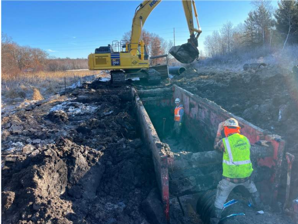
Photo #1: Checking the centerline of pipe to make sure it's lining up with the manhole - Jan 29, 2024, 9:35 AM
