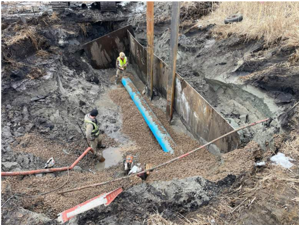
Photo #3: Connecting bored force main from under Highway 10 with the force main to go to the outlet structure - Jan 30, 2024, 12:17 PM
