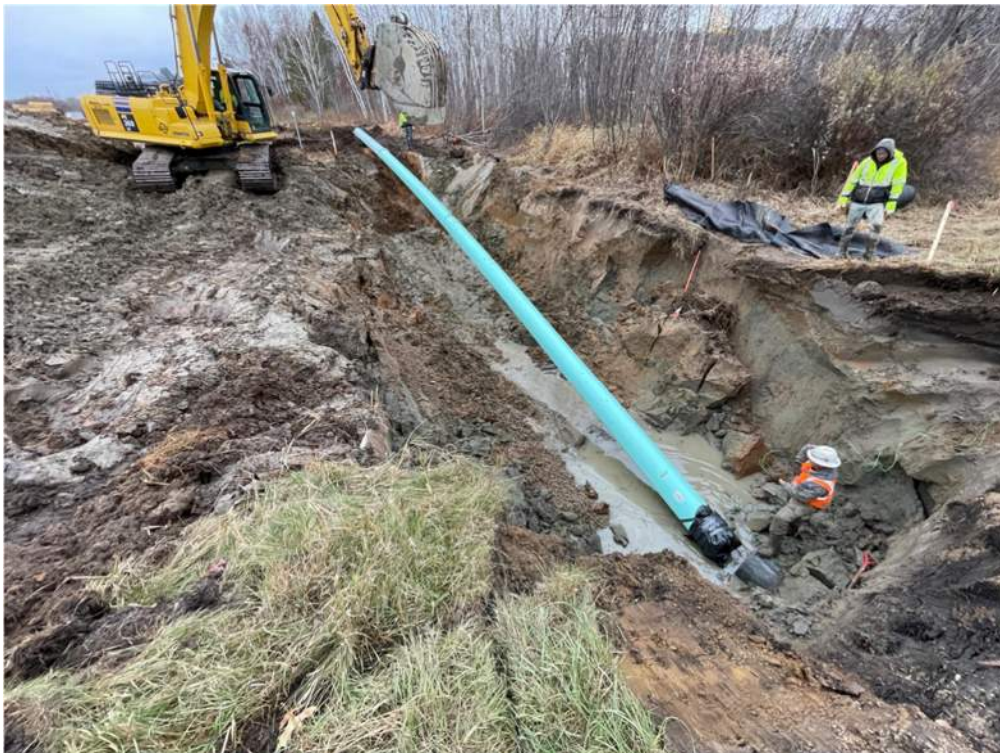
Photo #2: Lowering force main pipe to guide it into carrier pipe. - Nov 6, 2023, 3:58 PM
