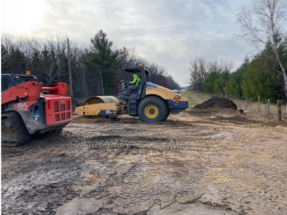
Photo #5: Compacting sub grade that will be under the repaved portion of Atlantic Road - Nov 8, 2023, 9:26 AM
