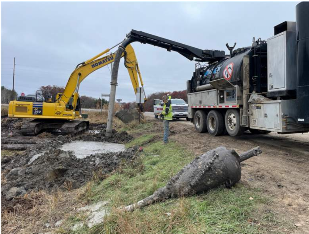
Photo #4: Vacuum truck taking care of excess mud from pulling the carrier pipe back through the bored hole. - Nov 7, 2023, 10:39 AM
