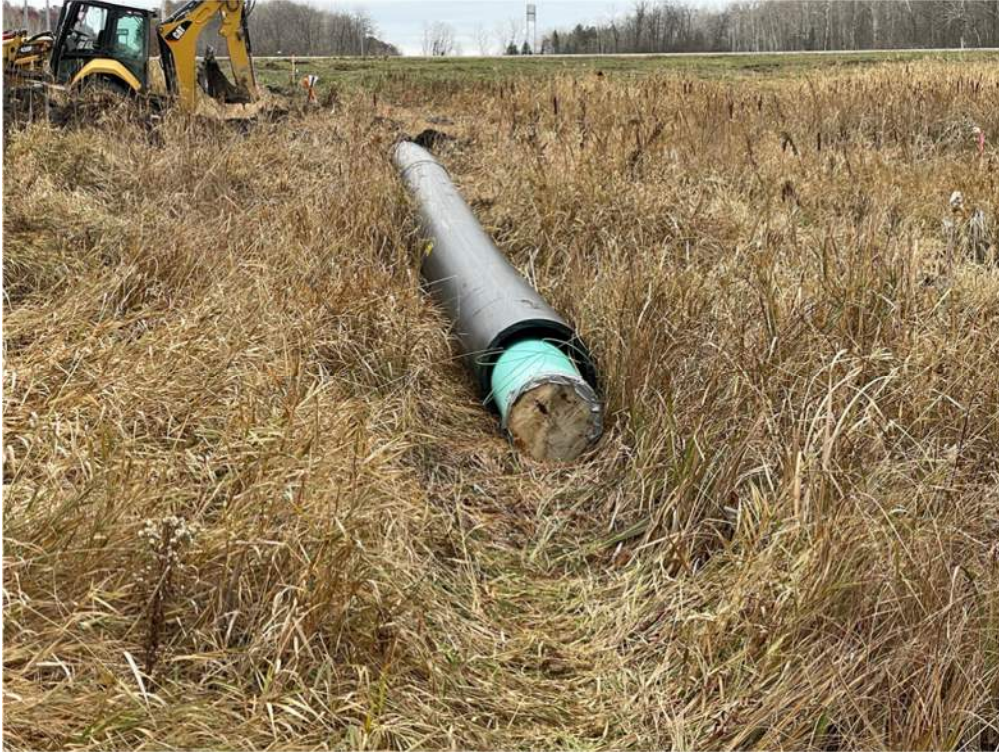
Photo #3: Carrier pipe and force main pipe ready to be pulled through the bored area under Highway 10. - Nov 7, 2023, 9:45 AM
