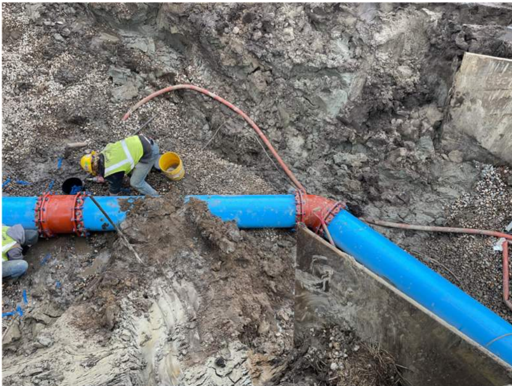
Photo #6: Bored force main from under County Road 203 and Highway 10 being joined together - Nov 8, 2023, 2:16 PM
