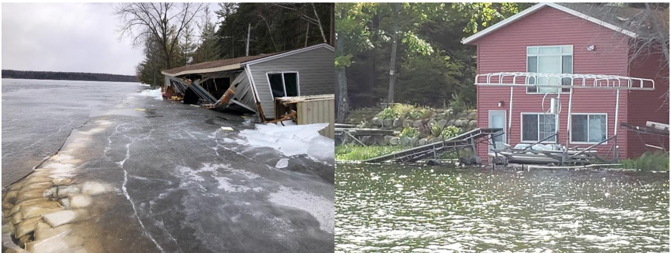
Cabin destroyed (and now removed). Many homes have water in their lower levels and basements.
