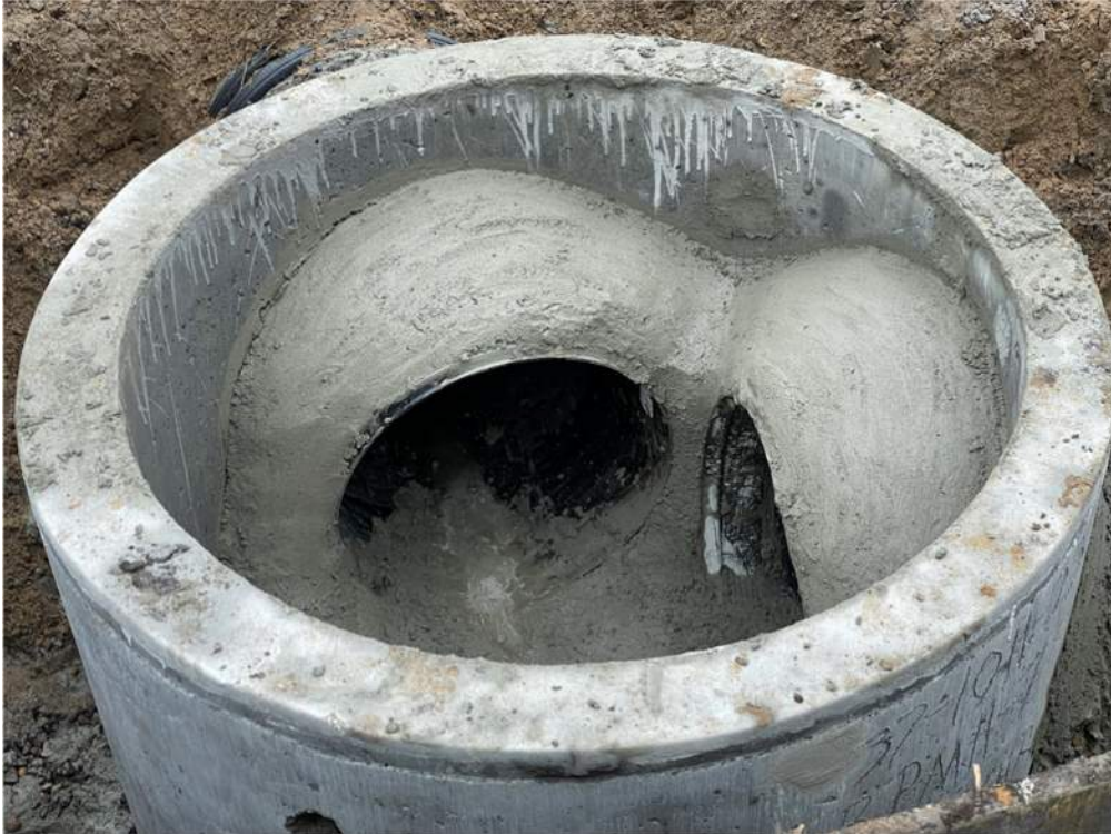
Photo #4: Gaps sealed with concrete around pipes and manhole bottom - Nov 21, 2023, 9:41 AM
