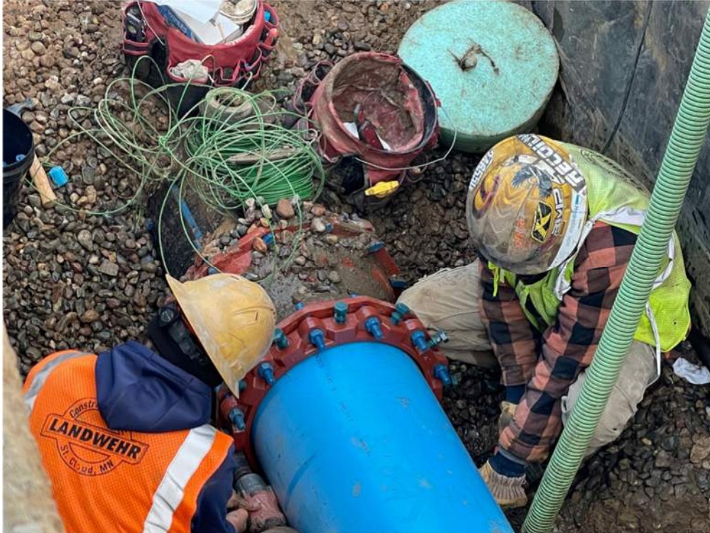
Photo #6: Installing reducer before preparing it to be wrapped in polyethylene film - Nov 22, 2023, 8:20 AM
