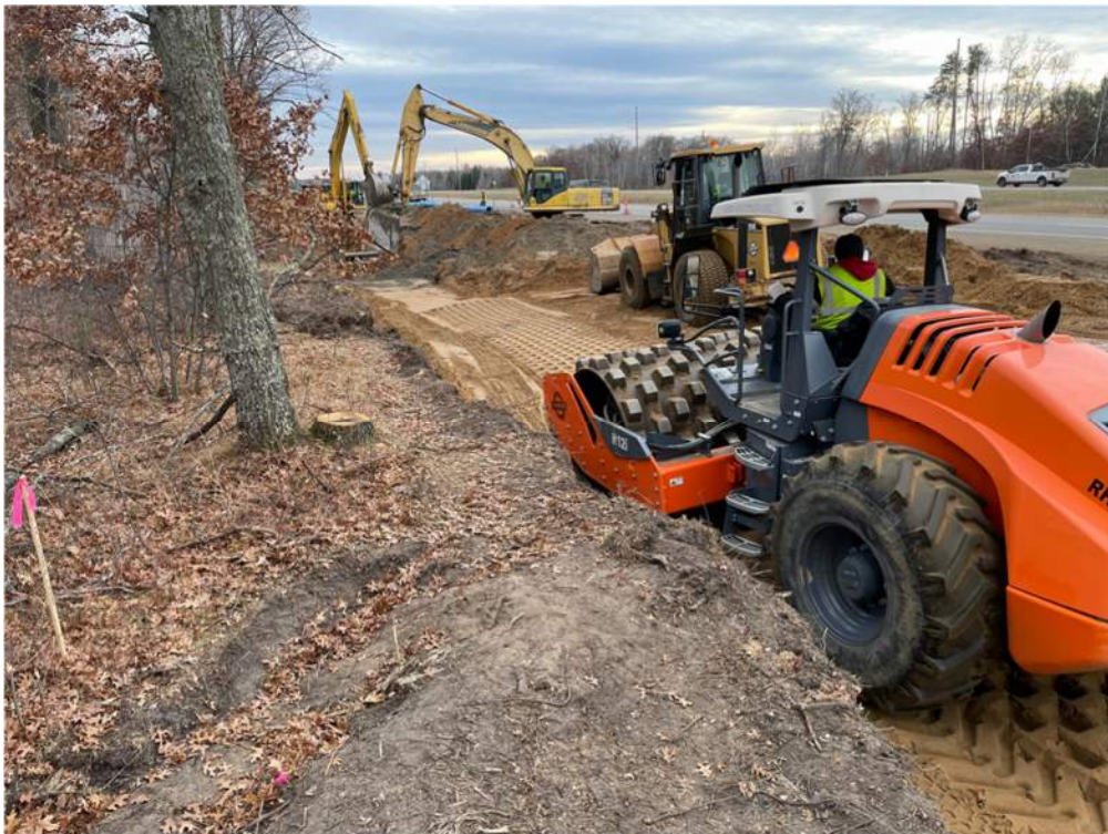
Photo #9: Compacting backfill over force main pipe with sheepfoot roller - Nov 22, 2023, 2:50 PM
