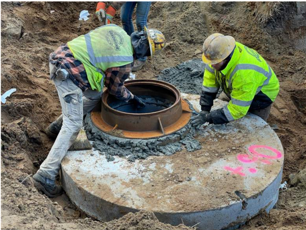
Photo #5: Installing concrete ring and metal frame to finish the manhole at the desired elevation - Nov 21, 2023, 10:22 AM
