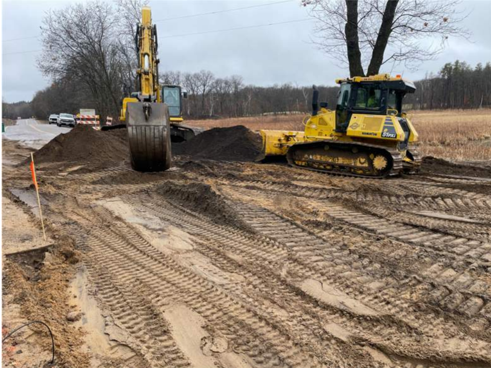
Photo #3: Scraping/pushing material closer to the excavator to be loaded and hauled out - Apr 8, 2024, 10:25 AM
