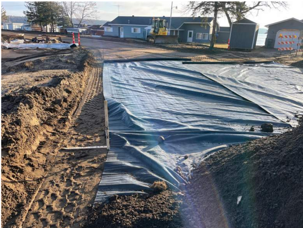
Photo #4: Getting geotextile fabric rolled out and ready on Aztec Road - Apr 9, 2024, 7:52 AM
