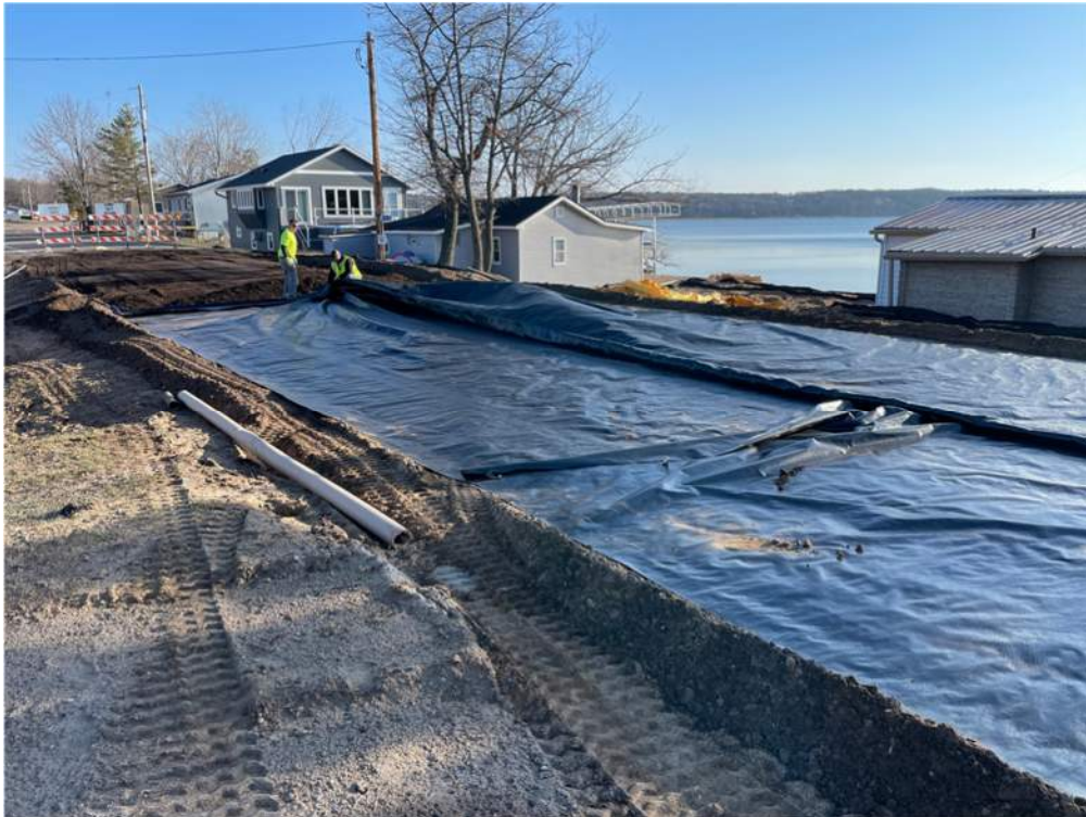
Photo #6: Laying geotextile fabric over the subgrade of Aztec Road - Apr 11, 2024, 8:10 AM
