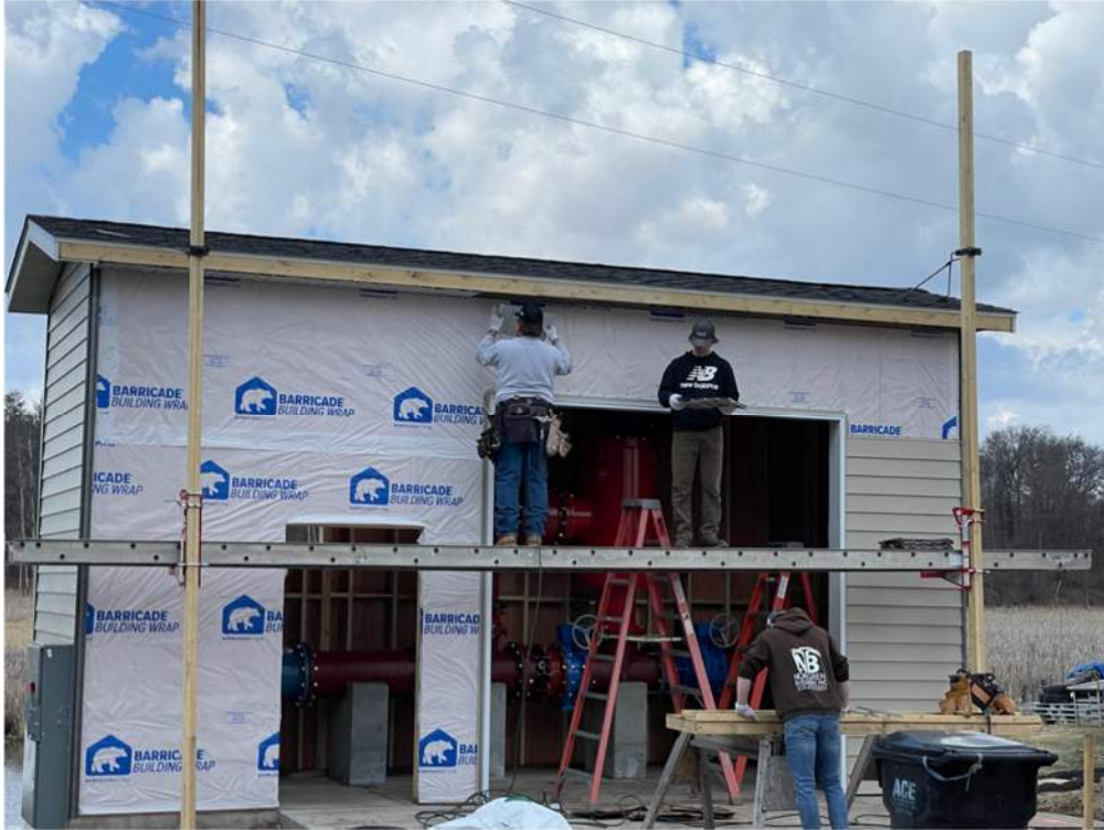
Photo #5: Installing the soffit pieces along the front of the pump house - Apr 9, 2024, 1:18 PM
