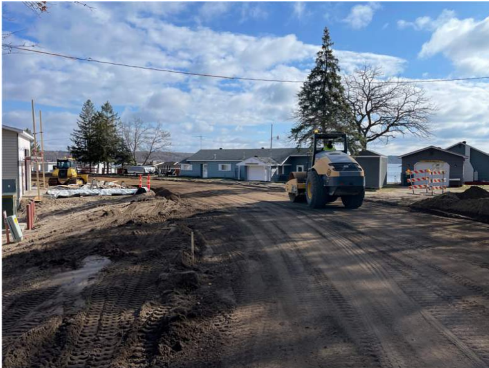
Photo #8: Rolling and compacting the aggregate base on Aztec Road - Apr 11, 2024, 9:44 AM
