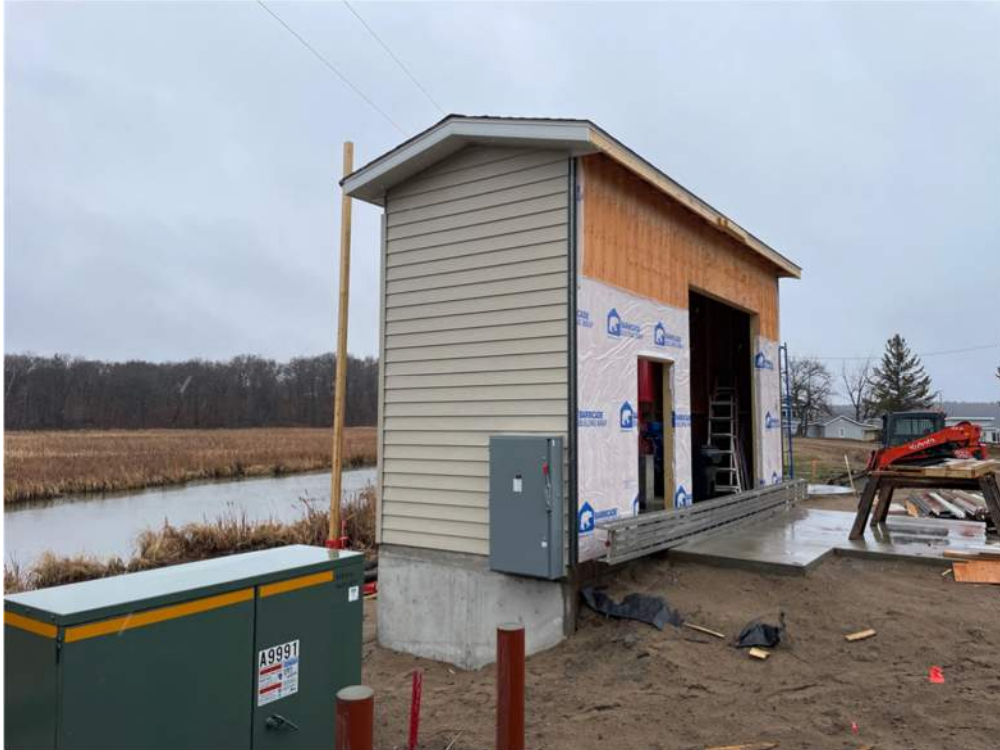
Photo #1: Siding, soffit, and fascia installed on the south side of the pump house - Apr 8, 2024, 8:04 AM
