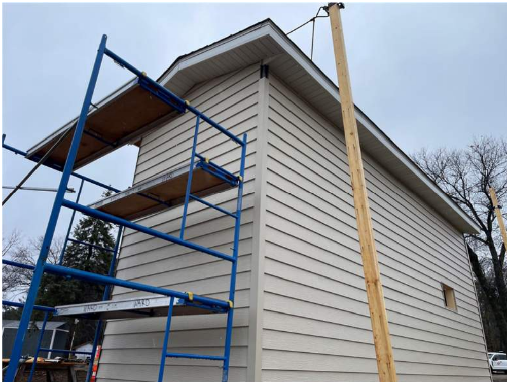
Photo #2: Siding, soffit, and fascia installed on the north side of the pump house - Apr 8, 2024, 8:05 AM
