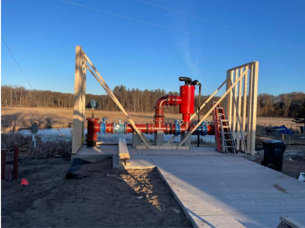
Photo #3: Two sidewalls of the pump house have been set - Mar 20, 2024, 7:57 AM
