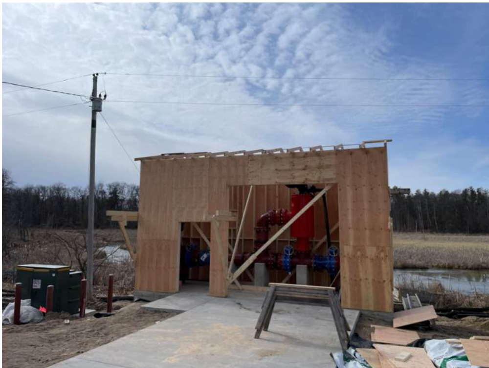
Photo #8: All plywood siding is on the structure walls and all trusses are nailed down - Mar 21, 2024, 3:15 PM
