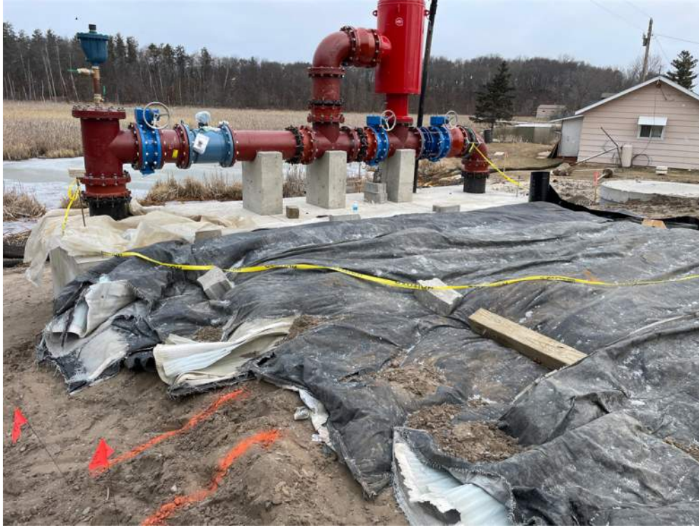
Photo #1: Concrete driveway heated with ground thaw unit and covered with concrete blankets - Mar 18, 2024, 7:53 AM
