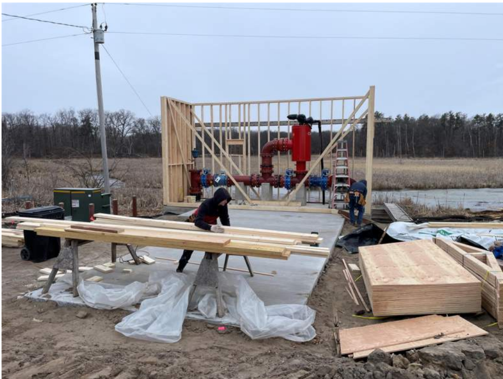
Photo #6: Ward Custom Homes is continuing to construct the walls for the pump house - Mar 21, 2024, 8:58 AM
