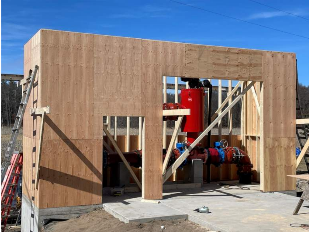
Photo #7: All four walls are up, and plywood is being added - Mar 21, 2024, 1:20 PM
