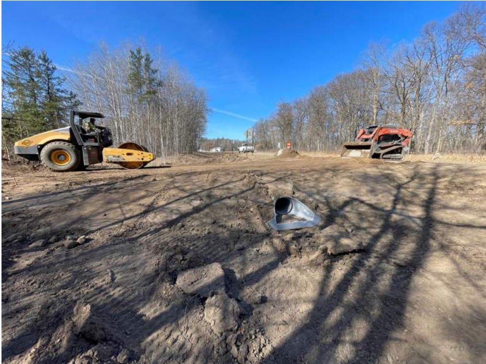
Photo #4: Rolling and compacting the sub grade below the driveway along Aztec Road - Mar 20, 2024, 11:44 AM
