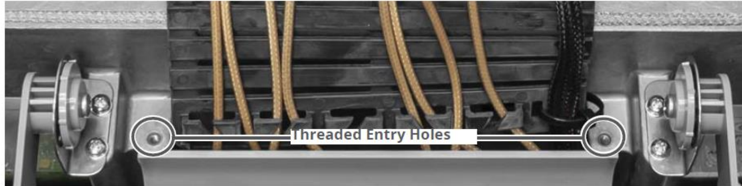
Installed Cable Shield
