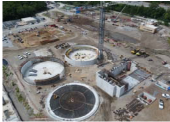
Wastewater Tomahawk Creek Wastewater Treatment Facility Leawood, KS
