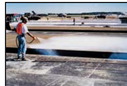
Wet burlap and white curing compound two different types of concrete curing.
