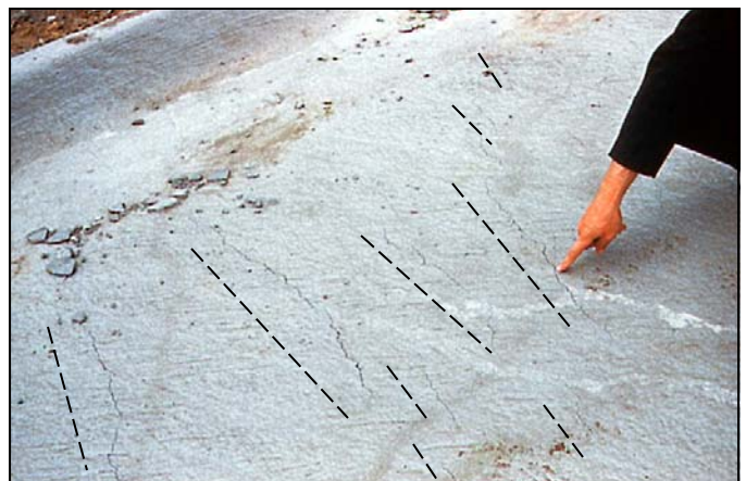
Plastic Shrinkage Cracks are typically associated with Hot Weather Concreting, or low air temperature, high concrete temperature, low humidity and high wind speed. These are often identifiable by their parallel structure, as in the picture above.
