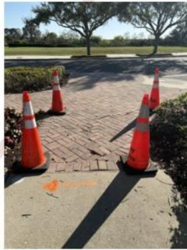
The pavers at The Independence Commons were beginning to come up from tree roots
