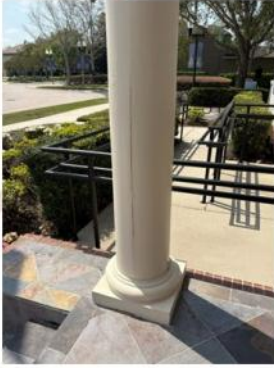
One of the pillars at The Town Square Residence Club was beginning to crack
